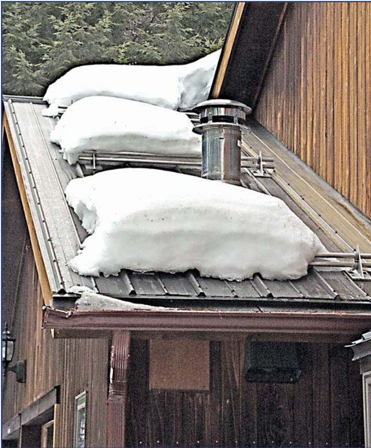
Figure 3 – Pipe-style snow guards create more of a barricade than pad-style snow guards.
