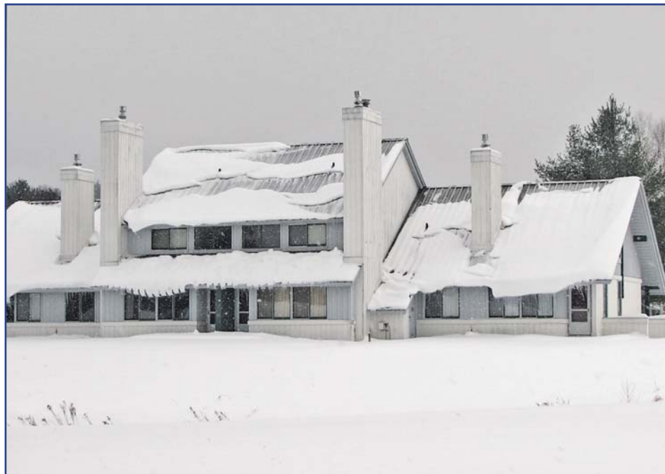
Figure 1 – Snow dumping from upper roof to lower roof, thus pushing snow off the lower roof above the door.
