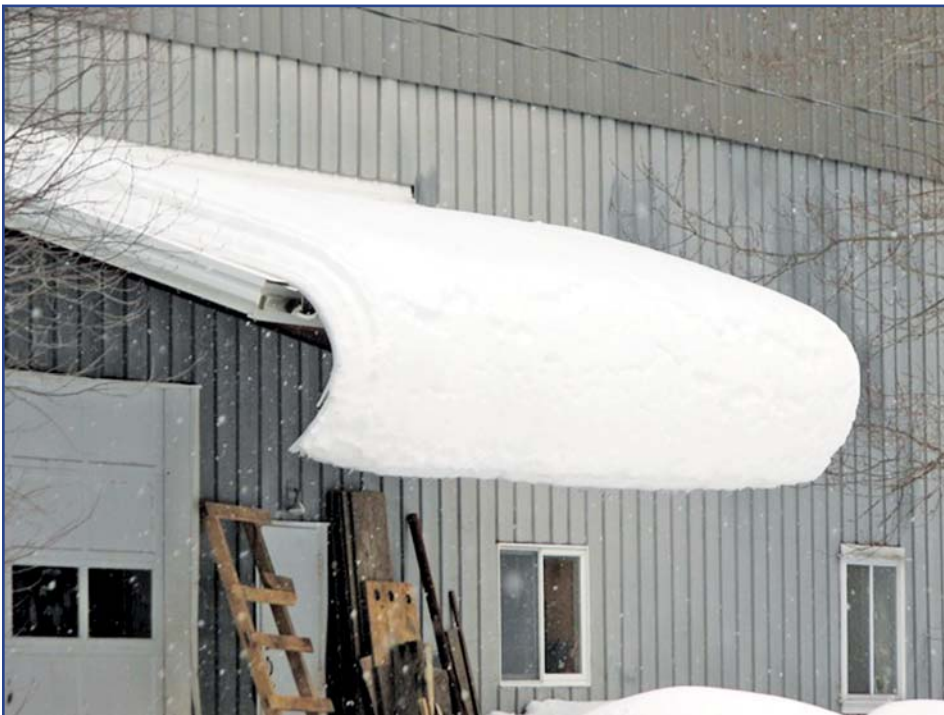
Figure 10 – This building, obviously with no snow retention devices, shows the typical “creep-and-curl” phenomenon.
