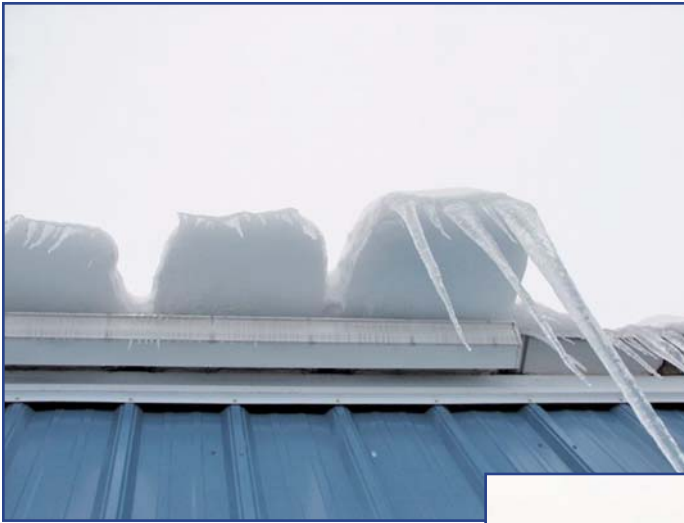
Figure 8 – Snow crept over the eaves as much as 18 inches on Alpine SnowGuard’s own building in Morrisville, VT.
