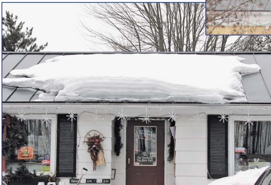
Figure 7 – Inadequate amount of snow guards above a door cause buildup of snow and get torn off each year.
