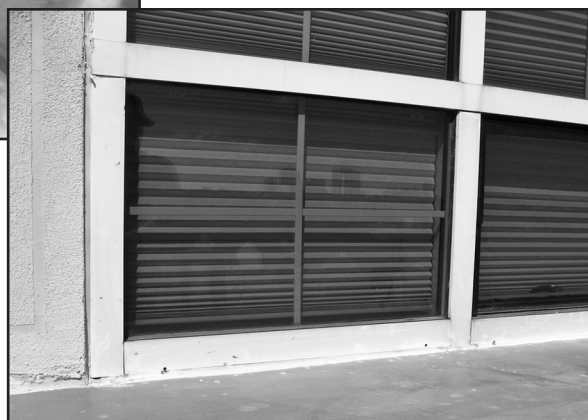
Figure 6 – Perimeter curtain wall sealant installed from adjacent cladding to snap cap of system.
