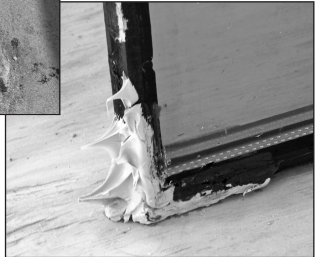
Figure 7B– View of insulated glass-unit corner after deglazing condition shown in Figure 7A.
