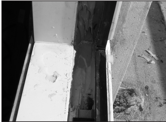
Figure 7A – Excessive sealant placed at the sill-to-mullion joinery.
