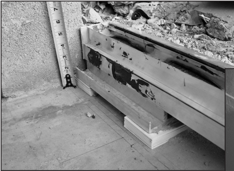
Figure 3 – Excessive shimming at unitized-system starter sill to accommodate concrete tolerances.
