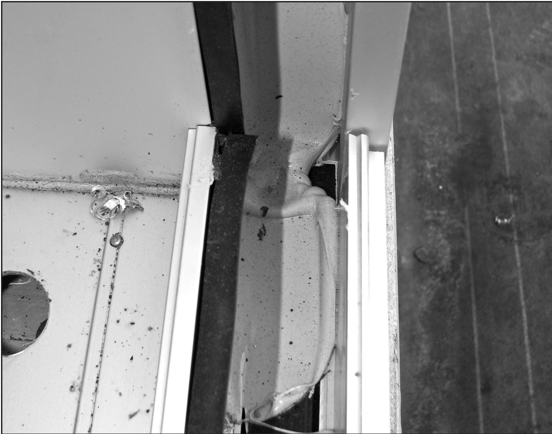
Figure 14 – Improperly tooled sealant at metal-to-metal joinery resulting in a large void.
