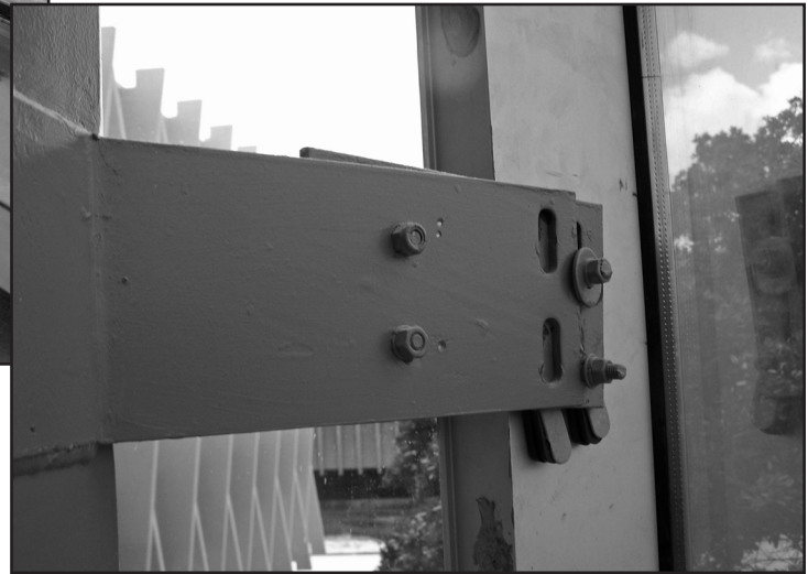
Figure 4 – Improvised wind clip at corner mullion to compensate for out-of-tolerance steel erection.
