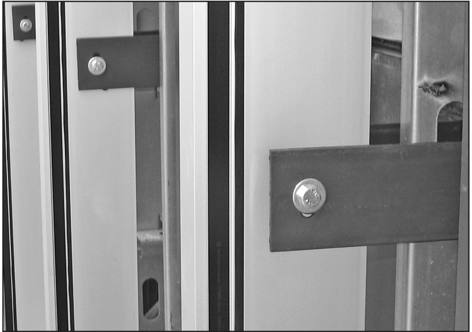
Figure 12 – Two adjacent wind clips, one with anchor at top of the slotted hole and one at base.
