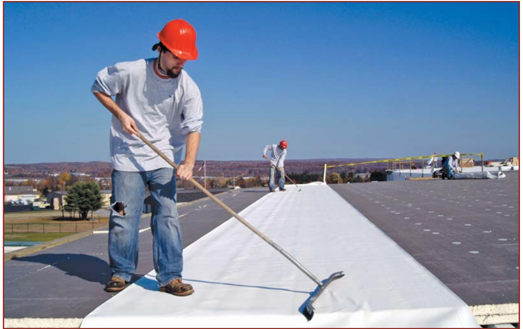
Photo 2 — Applying pressure to the membrane with a broom removes trapped air and increases contact points between the membrane and the substrate.
