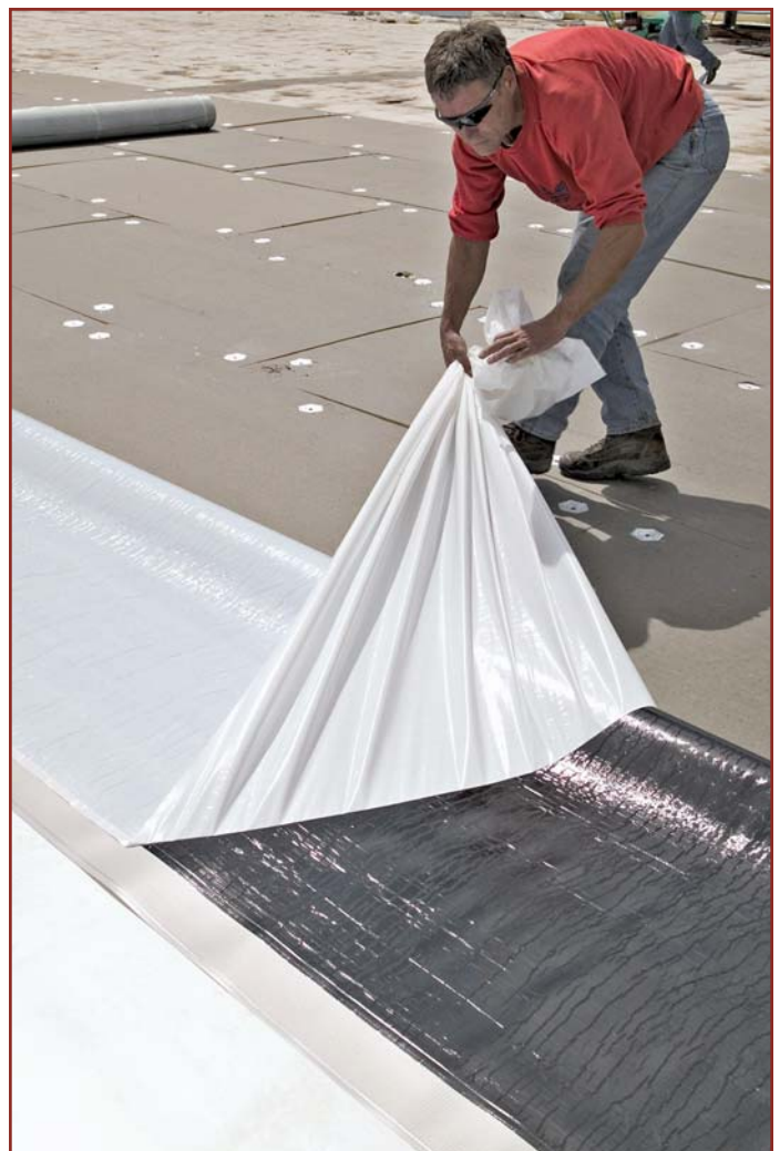
Photo 1 — Self-adhering TPO membranes are easy to install since the bonding adhesive is preapplied to the membrane. Peeling off the release liner exposes the hot-melt adhesive.
