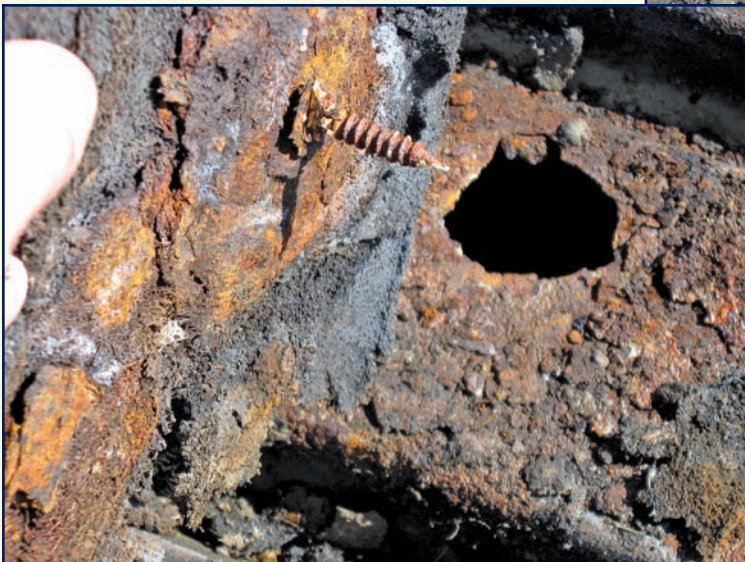
Photo 4 — The fasteners and plates were severely attacked.
