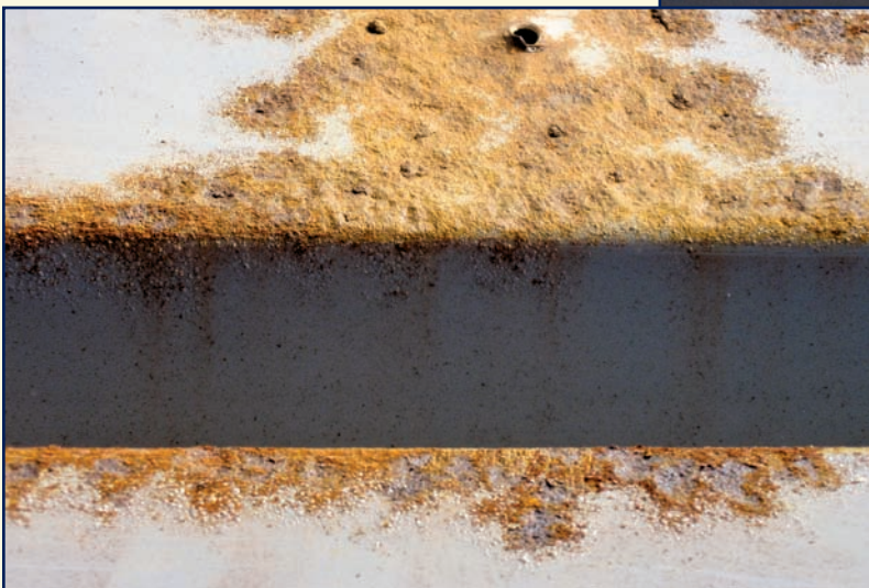
Photo 7 — A close-up of Photo 6 shows pitting and scale are developing. This was a former plate-and-screw location; the condition appears to accelerate at these locations.
