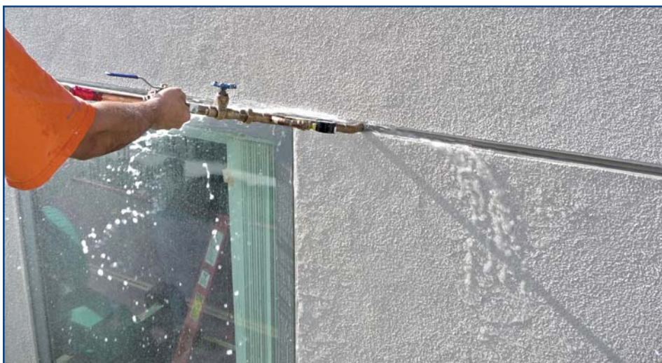
Photo 4 — Field water testing of #40 drift joints caused leaks. After remediation by installing sealant, subsequent field water testing did not result in leaks.
