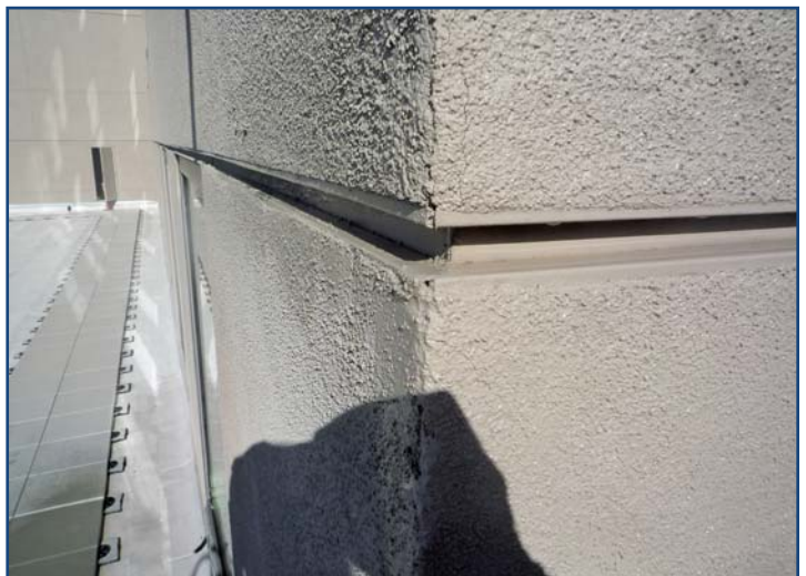
Photo 6 – Water leakage was occurring universally at the building interiors at the outside corners. This view shows the painted joint and stucco. The paint did not effectively seal the joint from water accumulating in the lower joint pocket and leaking out at the butt edges—first onto the WRB and eventually into the interior.
