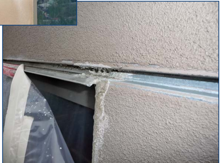
Photo 3 – Horizontal #40 drift joint intercepts water running down the stucco, which then flows back into the joint and into the pocket of the lower accessory. Note that stucco against the metal jamb flange is actually trapping moisture, which is behind it in the drift joint lower pocket. Problems also exist with the upper stucco being able to weep effectively.
