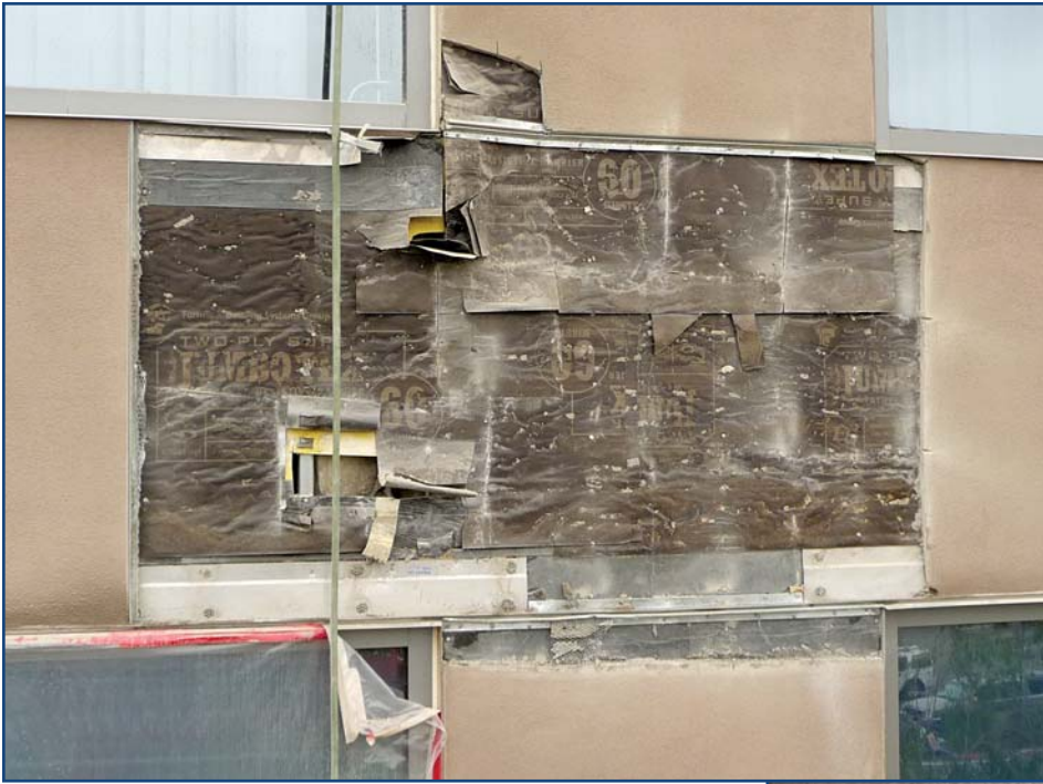
Photo 2 – This photo shows the typical drift joints (along the top of the windows in the lower portion of the photo) terminating at the window jambs and forcing moisture into the WRB, leading to uncontrolled ingress of moisture behind the stucco and leakage into the interior during heavy rain.
