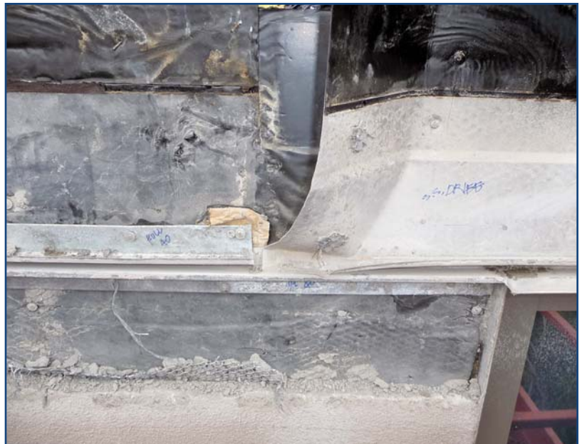
Photo 1 – Note the exposed termination of the lower pocket of the #40 drift joint against the window jamb metal flange. It is unsealed and will drain water that is trapped in the lower pocket into and down the jamb WRB. Water was leaking into the building at the window perimeters during significant rain and leaked from spray testing.
