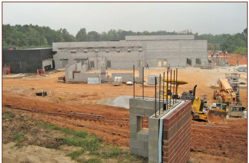
Figure 10 – Loose insulation blocking cavity.
