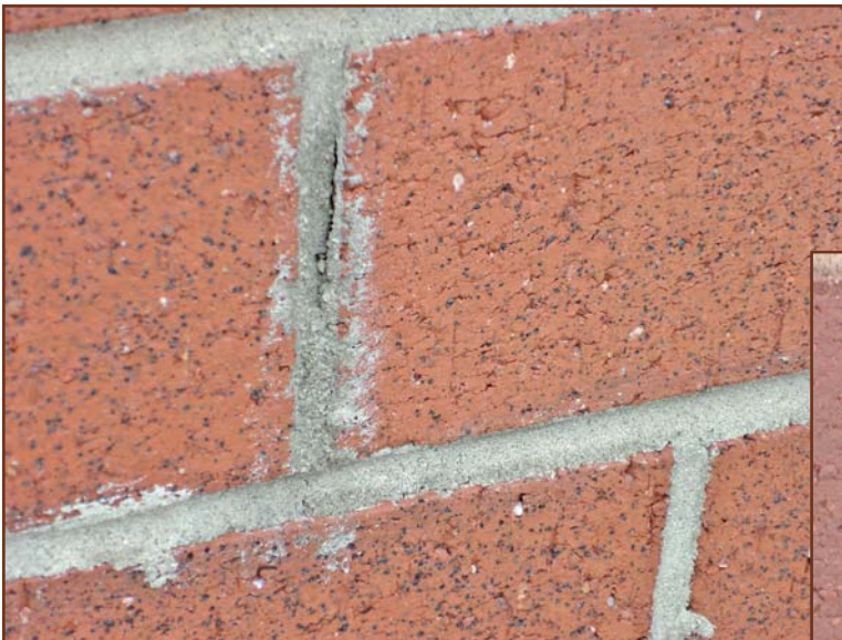
Figures 6A – Shrinkage cracks in mortar joints.
