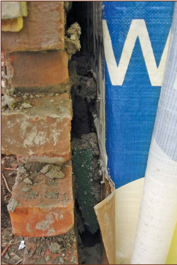
Figure 9 – Cavity impacted with mortar droppings.
