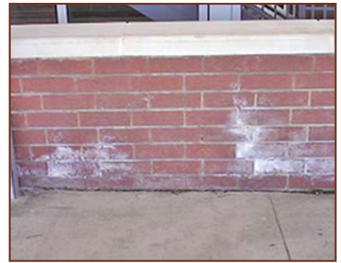
Figure 8B – Crystallized efflorescence.
