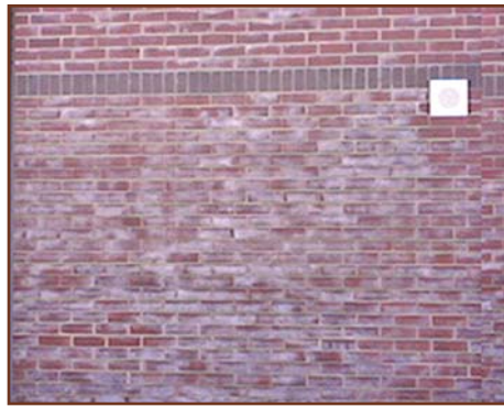
Figure 8A – Powdery efflorescence.
