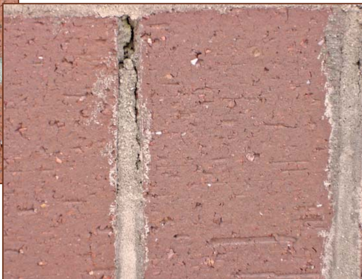
Figure 6B – Weak Bond in mortar joints.
