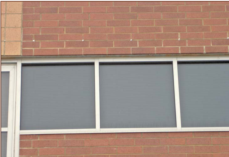
Figure 11 – Improperly located weeps.
