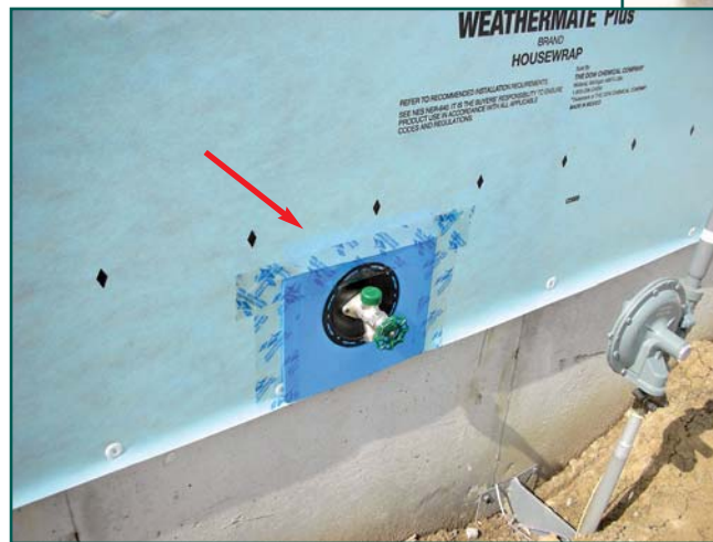
Photo 24 – Penetrations should be flashed and properly integrated with the house wrap (WRB).
