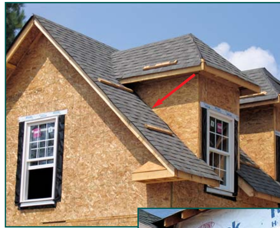
Photo 16 – Missing step flashing.
