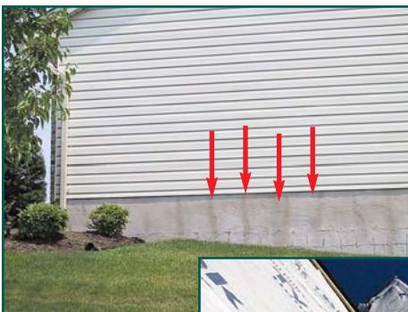
Photo 18 - Vinyl Siding Drainage
