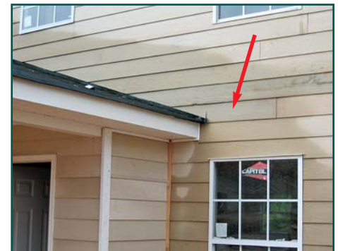
Photo 7 – Moisture at roof/wall intersection.
