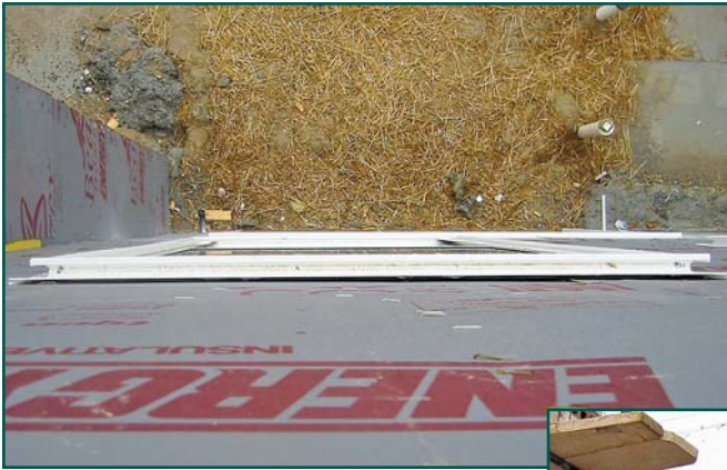
Photo 30 – Note the gap between the nail fin and the sheathing.
