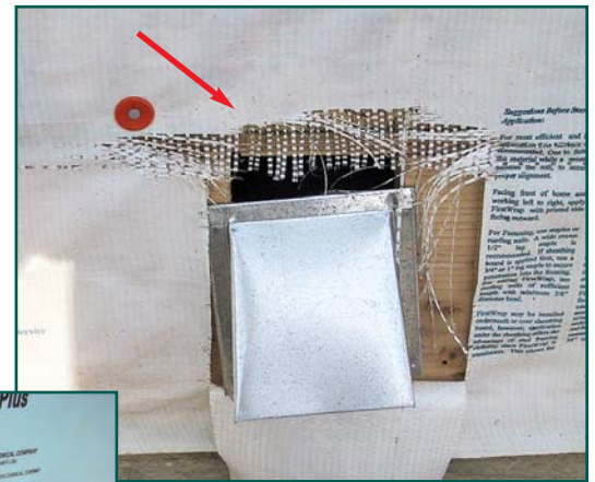
Photo 23 – WRB at vent should be flashed.
