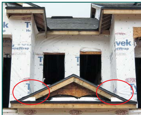
Photos 2 - Roof sloping into walls.
