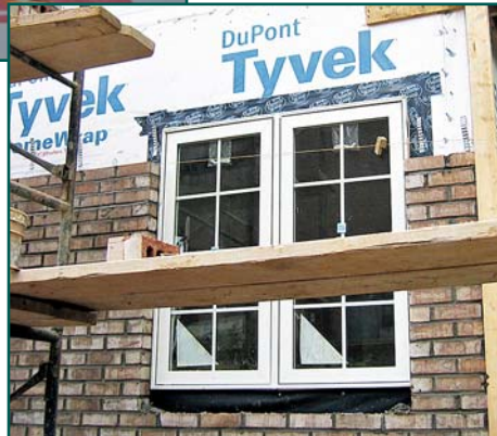
Photo 31 – Improper head flashing.
