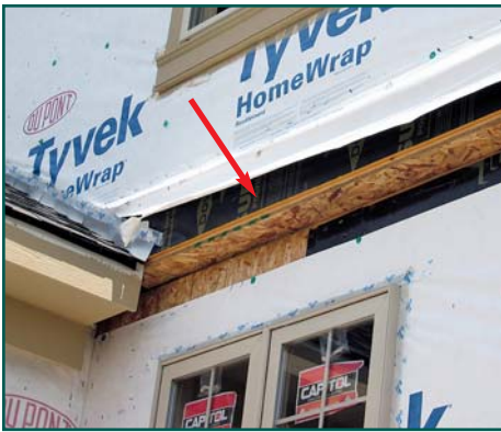
Photo 8 – Hole in water-resistive barrier (WRB).
