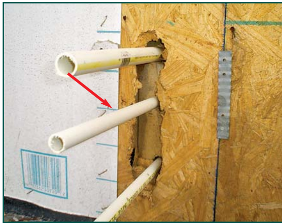
Photo 21 – No flashing around pipes.
