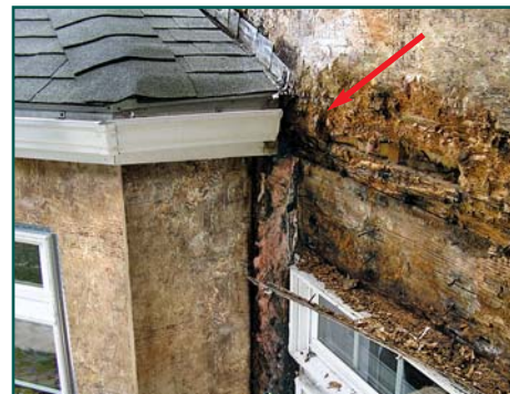
Photo 6 – Damage at roof/wall intersection.
