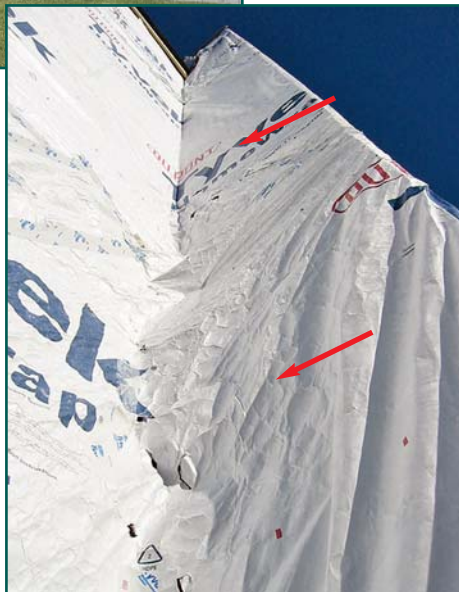
Photo 19 – Rips and gaps in WRB.
