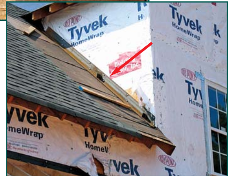
Photo 17 – Missing counter flashing.
