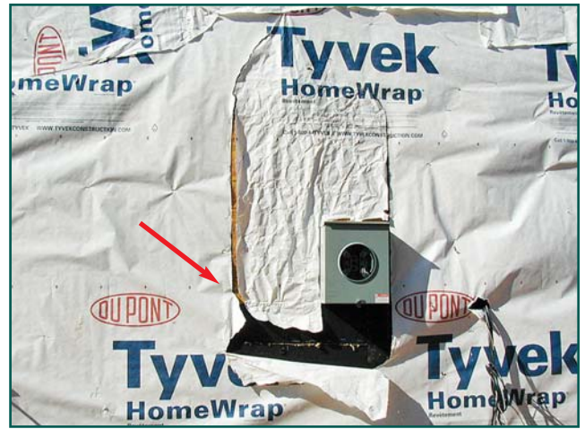
Photo 22 – Poor detailing at electrical meter.
