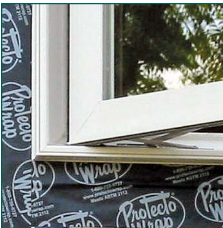
Photo 32 – Improper sill flashing.
