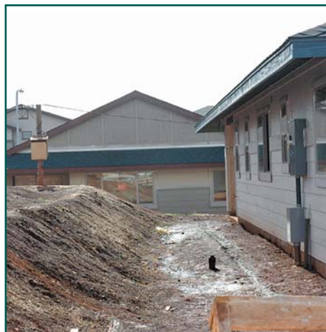
Photo 33 – Poor drainage design.
