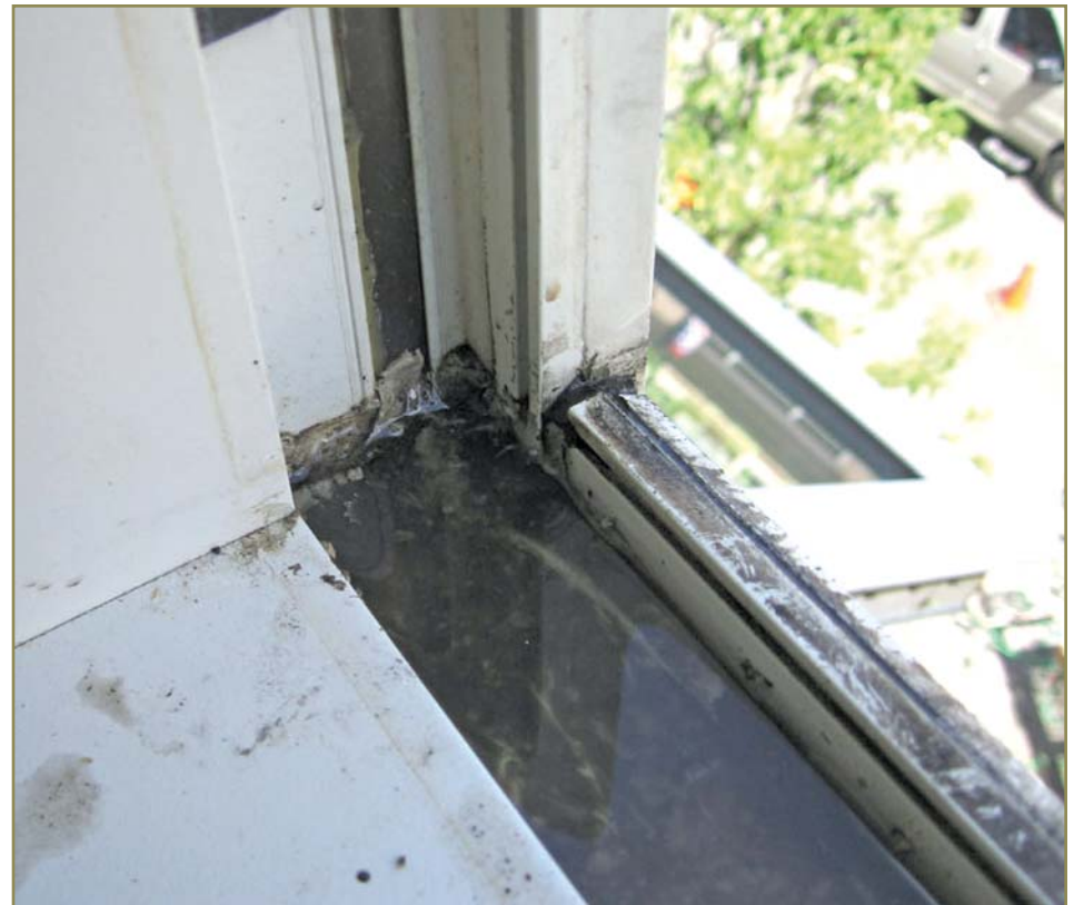
Photo 2 - Water ponding in curtain wall.
