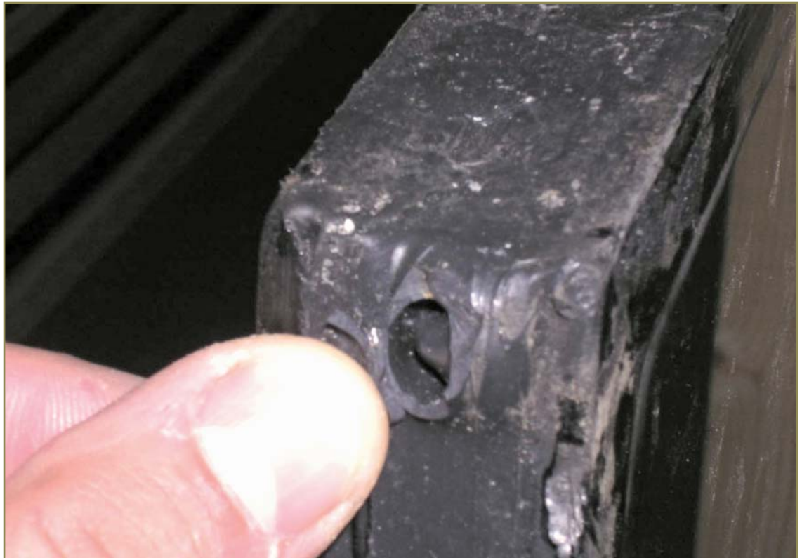
Photo 12 - Open blister in silicone secondary seal at the corner of an IG unit.
