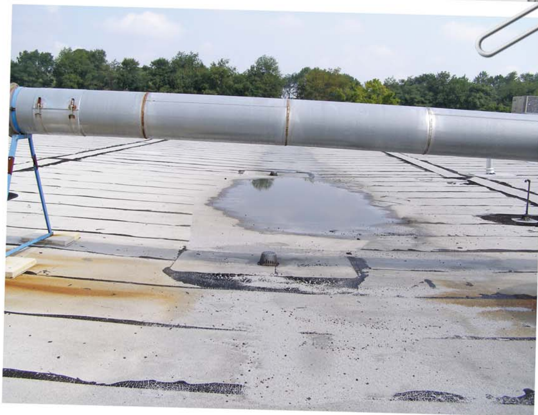
Ponding water in valley line before resloping with SPF.
