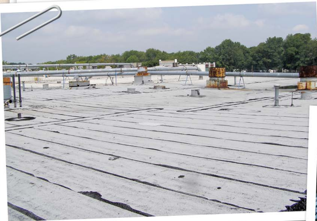
Field of roof before restoration.
