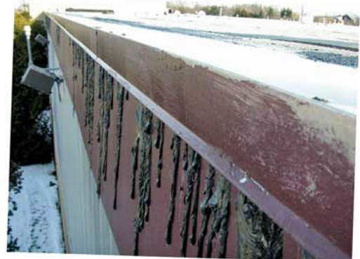
Coal tar seeping over roof edge.
