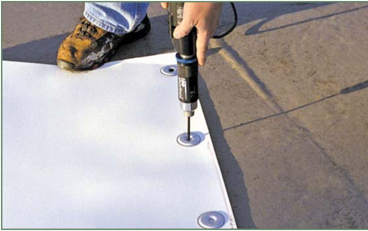
Photo 1 – SPRI investigated the role that fastener corrosion could play in roof failures and whether or not metal fastener corrosion in treated lumber is an issue. (Photo courtesy of GAF, Wayne, NJ.)
