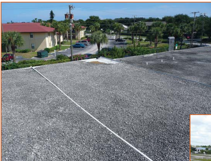
Figure 5 – Typical minor scour (Roof No. 16).
