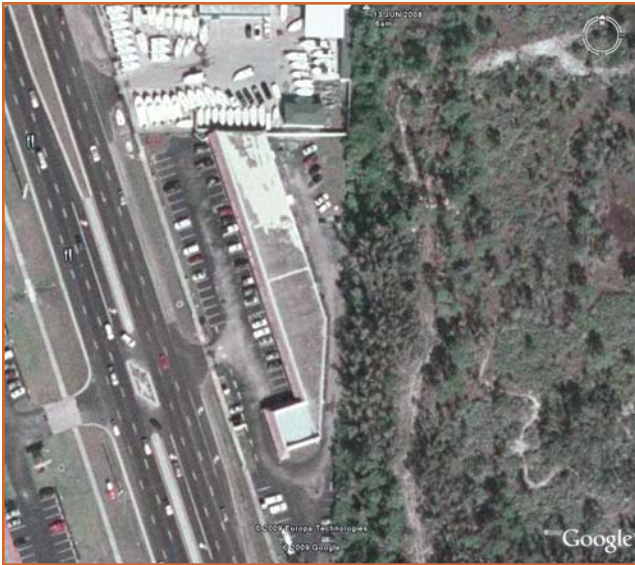
Figure 8 – Roof No. 13 exhibited aggregate loss. The roof had no parapet on the side facing Exposure C. Aggregate loss was from the northern half of this roof. Photo courtesy Google Earth.
