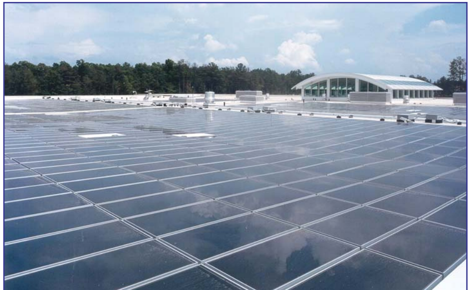
Photo 5 – The EPA’s Computer Center handles a massive quantity of data processing equipment. The output from the solar collectors offsets approximately 5% of the building’s energy consumption, which is estimated to be approximately twice that of a conventional office building of equivalent size, due to the large demand from data processing equipment. Photo courtesy of the EPA.
