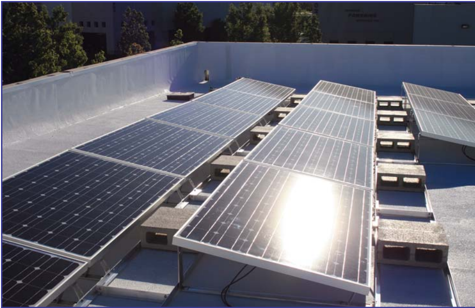
Photo 2 – A cool roof as an integral component of a solar installation enhances reflectivity and other benefits, such as cooling a building’s interior and helping to improve the operation and efficiency of the photovoltaic system. Solar systems work best at temperatures below 90°F. If temperatures exceed 110°F, the solar power output can be reduced by as much as 50%. Photo courtesy of Coat’N’Cool.
