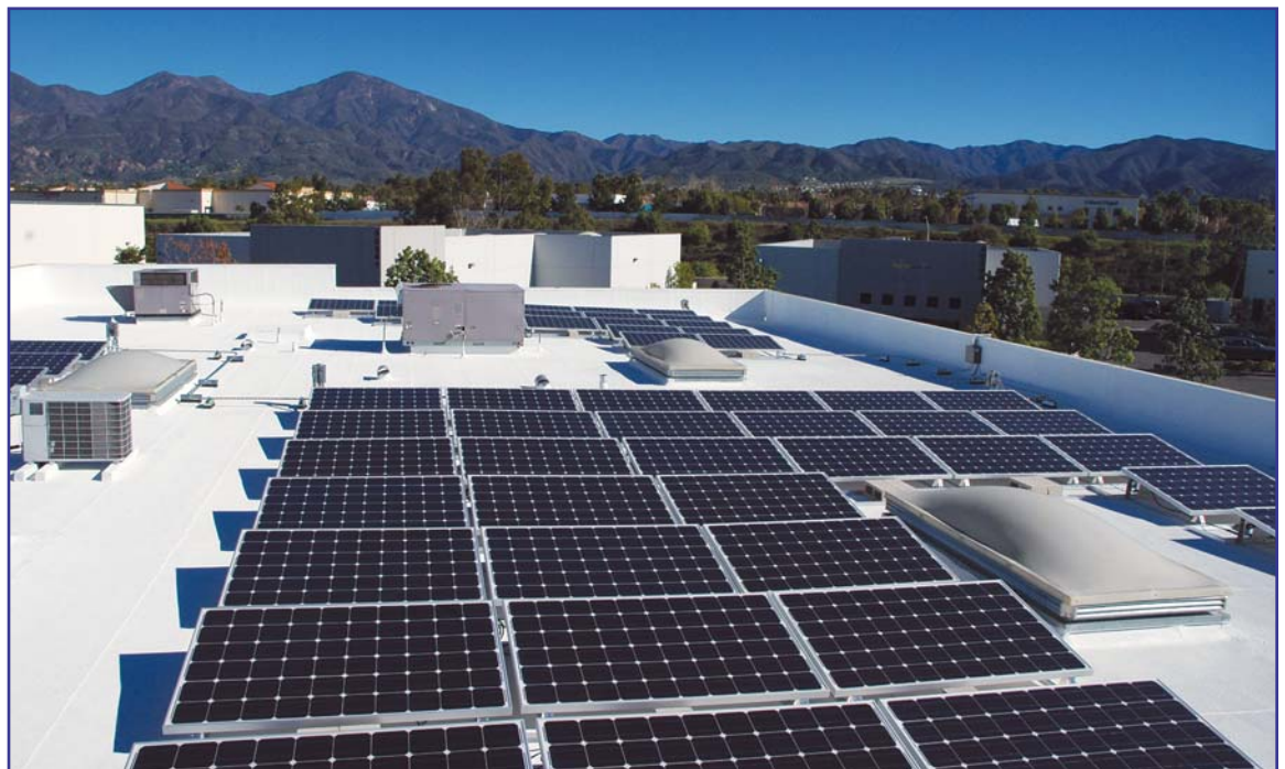
Photo 1 – One solar installation company that has embraced the marriage of solar panels and cool roofs is Advanced Powering Services, Inc., of Rancho Santa Margarita, CA. The company has installed a cool roof/solar panel beta test site on the roof of an industrial building. Photo courtesy of Coat’N’Cool.
