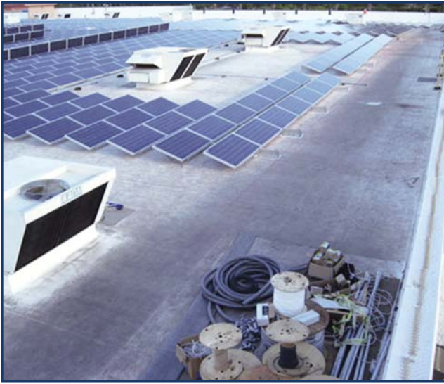
Photo 1 – New TPO roof damaged during PV installation. Courtesy of Firestone Building Products.
