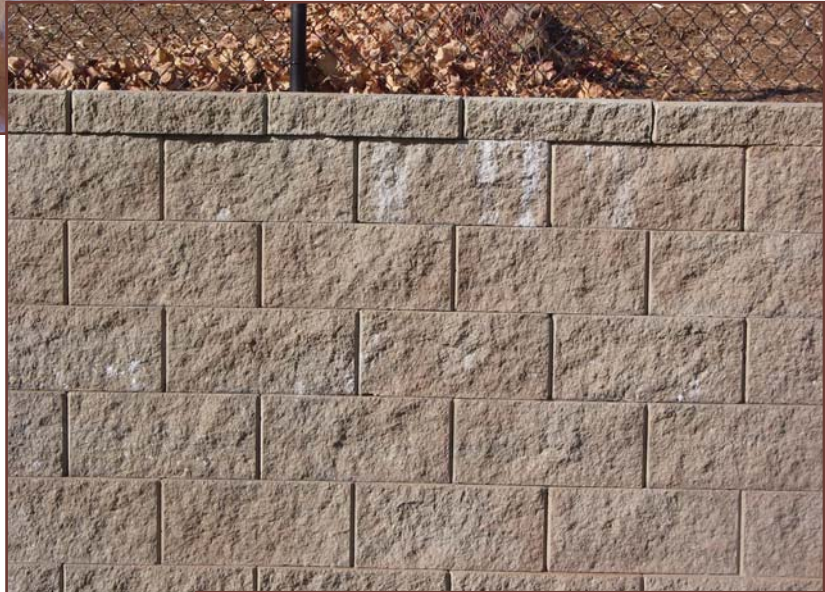
Figure 4 – Efflorescence caused by improper drainage and no waterproofing behind the retaining wall.
