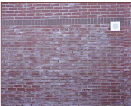
Figure 1 – Efflorescence caused by cold, damp weather. Very severe efflorescence can make masonry appear as if being observed through a frosted glass. The wall was clear by late spring.
