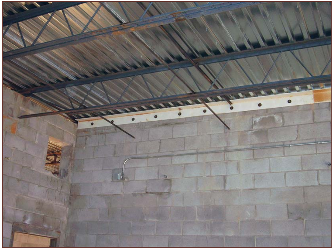
Figure 15 – New construction efflorescence from residual moisture that usually disappears after the building dries out.
