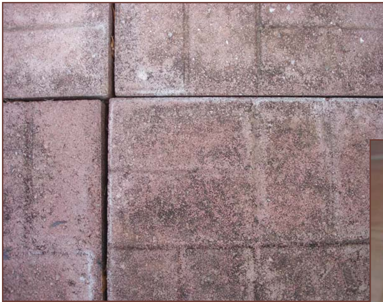
Figure 7 – Efflorescence mixed with traces of mildew on shaded concrete pavers caused by moisture migrating from unprotected base.
