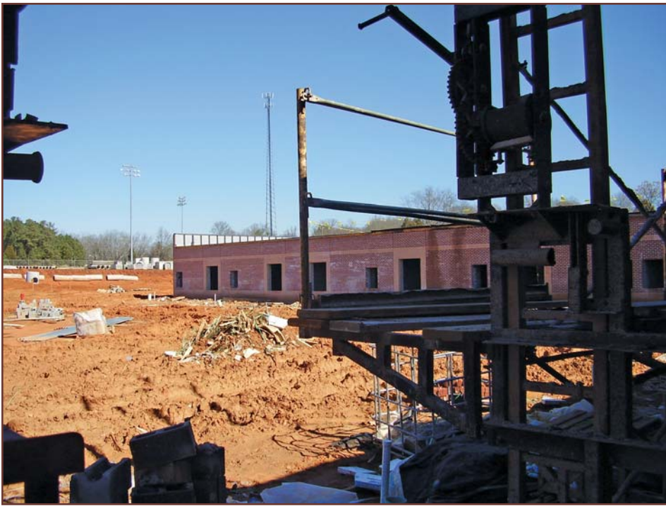
Figure 14 – New-building bloom during winter construction usually disappears after everything dries out, especially after the interior acclimates.
