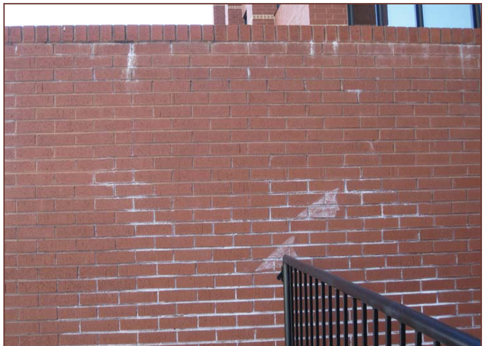
Figure 2 – Moisture migrating through the brick cap of a brick retaining wall produced traces of lime run and efflorescence.
