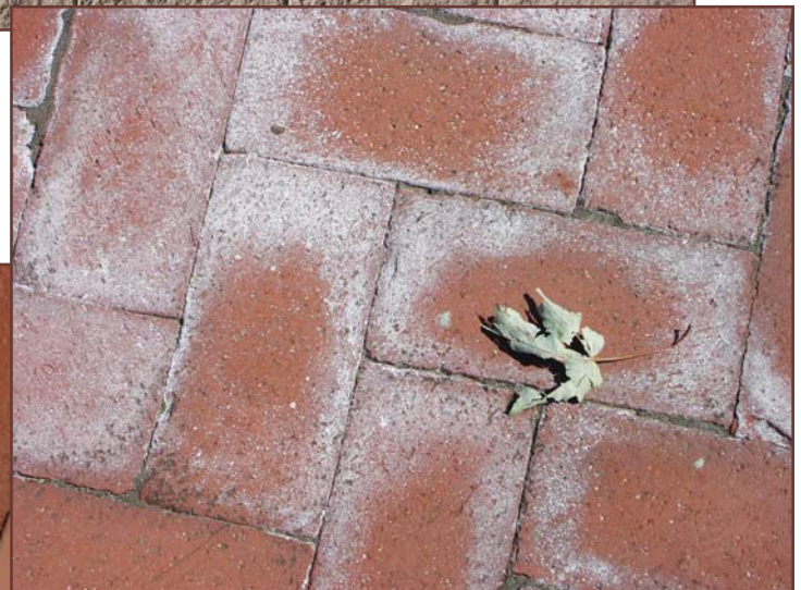
Figure 6 – Efflorescence on shaded clay pavers over an unprotected base.
