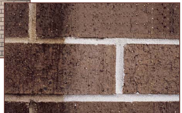
Figure 10 – Manganese metallic stain leaves its dark mark that often resembles tobacco stain. (Courtesy of PROSOCO.)
