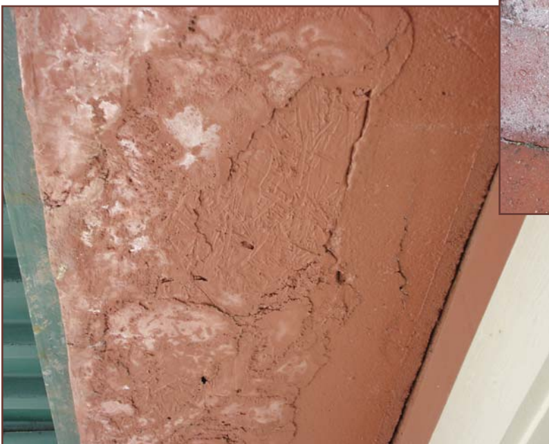
Figure 5 – An improper metal canopy tie-in directed moisture to the concrete lintel, causing efflorescence, spalling, and deterioration of attempted repairs.
