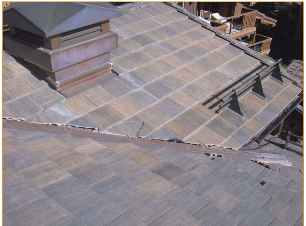
Photo 1 – Damage due to snow and ice accumulation in the valley area. The edge of the tile and the supporting valley flashing must provide structurally sound products in this area.
