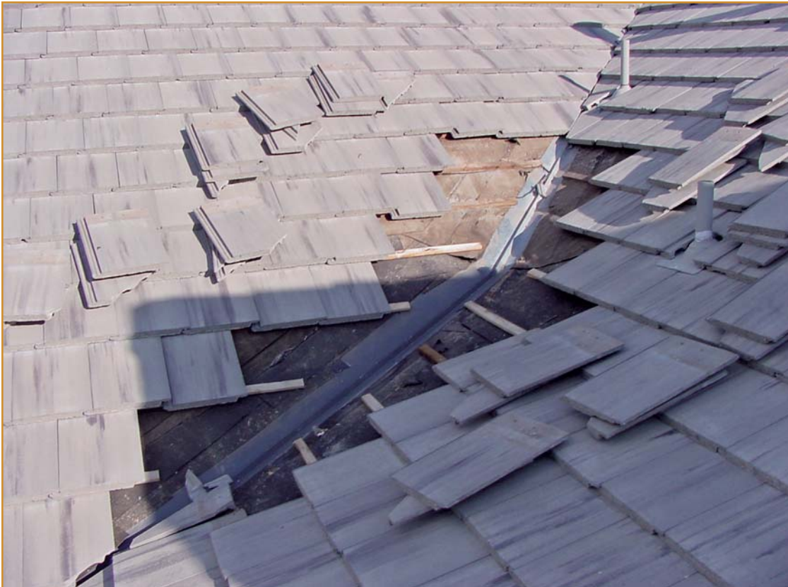
Photo 7 – This valley is constructed with horizontal battens that will trap debris. The use of a closed valley requires that tiles be removed in order to perform the required maintenance.
