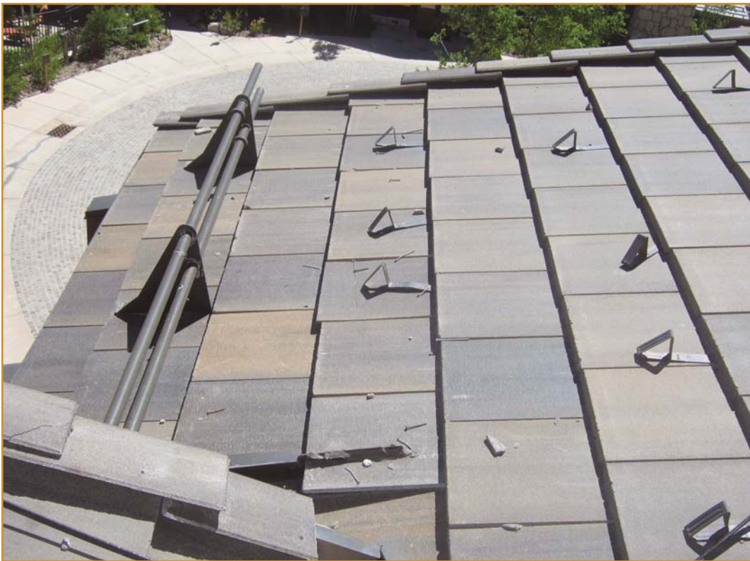
Photo 9 – Snow damage of the cleats and tiles due to build-up of ice and snow behind the retention bars. The clips do not have structural capacity to resist the loads imparted from the sliding ice and snow.
