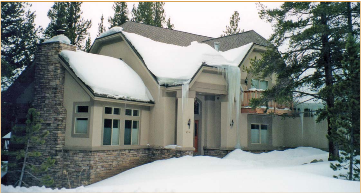
Photo 2 – Roof layout and an understanding of ice and snow accumulation are extremely important and should be fully considered by the design and construction team prior to applying the roofing and integrating the building veneers.
