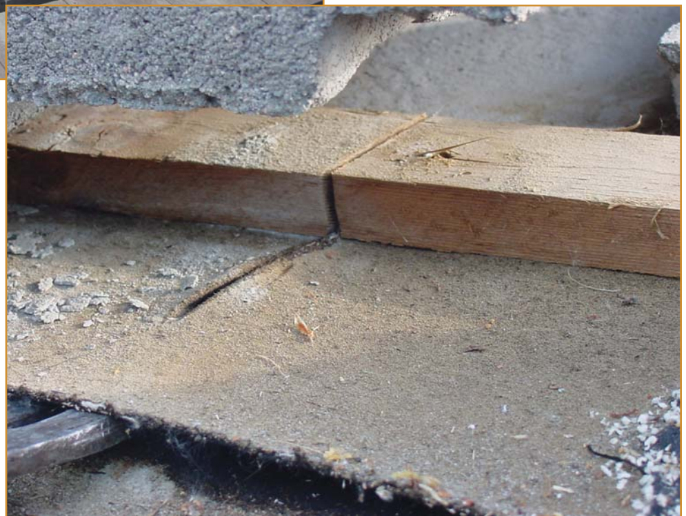
Photo 12 – Horizontal battens require that water drain to the slots. In order for that to happen, water must back up and work its way to the drainage slot. In the photo below, the slot appears to have been cut after the installation of the batts; this creates an opening in the roofing felts for the water to drain through. Vertical battens with the horizontal battens applied over the top are preferred over this type of installation because they create a direct and uninterrupted path to the edge of the roof.
