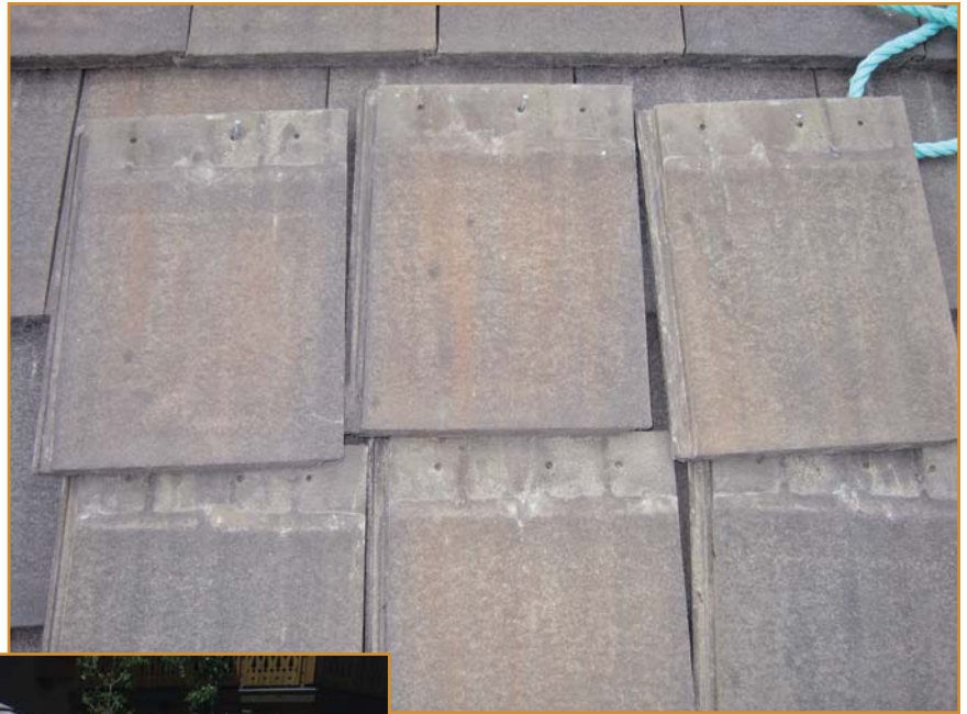
Photo 10 – The installer must determine the proper fastening and location. This as-built condition shows the nail size chosen and that there are missing nails in the tile roofing.
