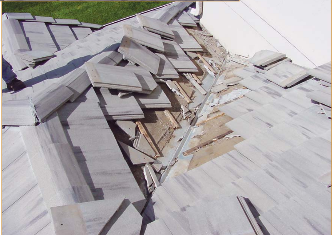
Photo 8 – Poor valley design by the architect is shown here. The design directs water into the vertical unit-demising wall and allows buildup of ice and snow against the cladding.
