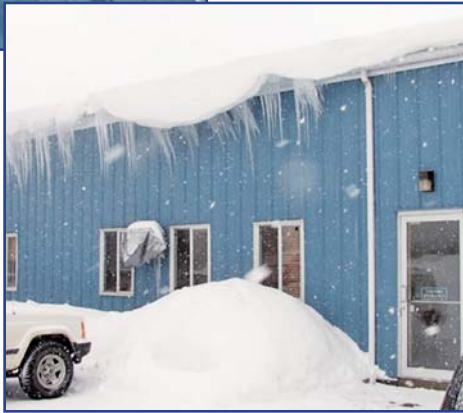
Figure 9 – Creep effect is witnessed on Alpine SnowGuard’s metal structure.
