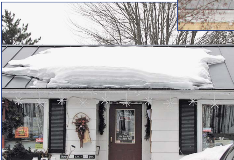
Figure 7 – Inadequate amount of snow guards above a door cause buildup of snow and get torn off each year.
