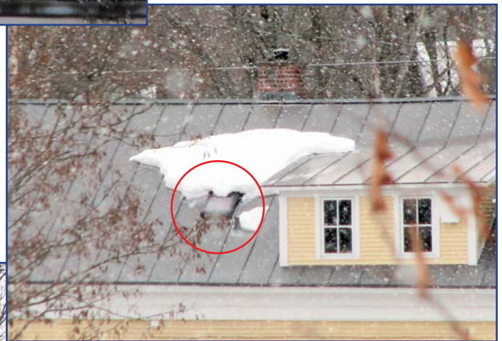
Figure 6 – Small skylight holds back an inordinate amount of snow relative to its size.
