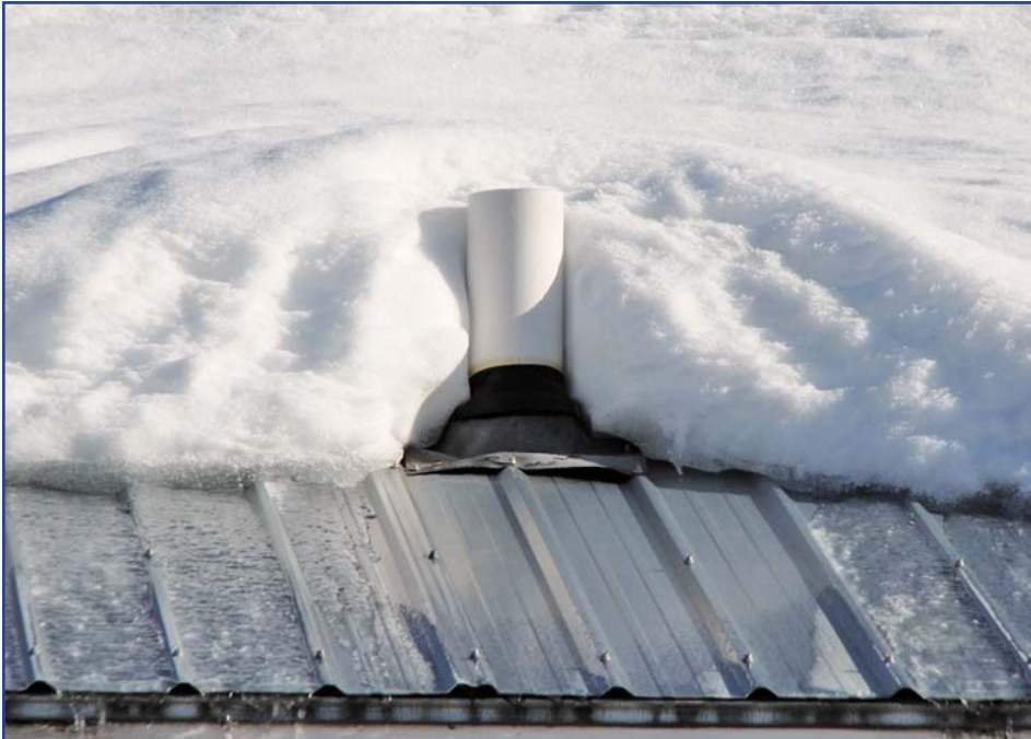
Figure 5 – Standard 3-in plumbing vent prevents snow from sliding off a metal roof.
