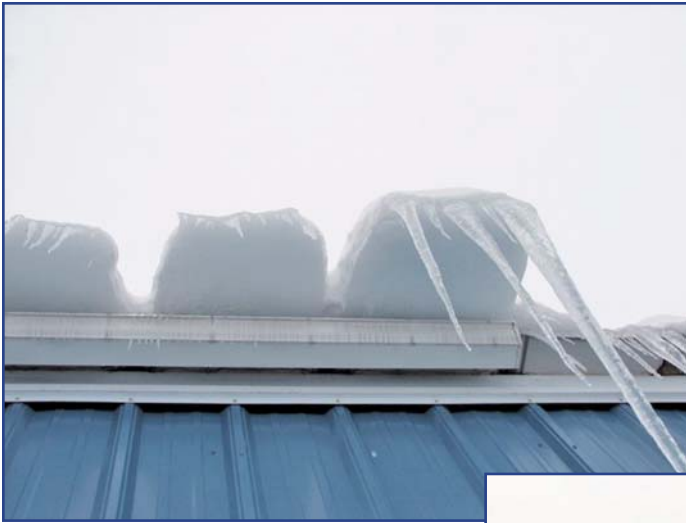
Figure 8 – Snow crept over the eaves as much as 18 inches on Alpine SnowGuard’s own building in Morrisville, VT.
