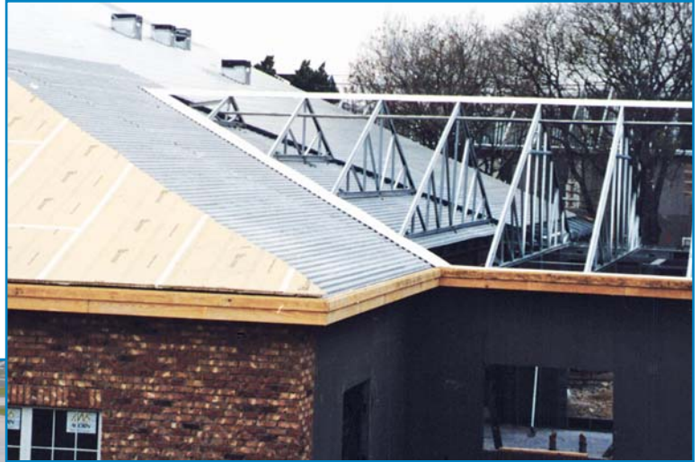
Photo 3 – Loadmaster nailable assembly over cold-formed framing with shingle application on an assisted-care living facility.
