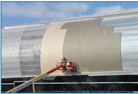
Photo 4 – Loadmaster insulated barrel roof assembly with standing-seam metal roof on an airport concourse.
