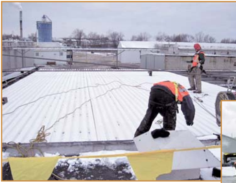
Photo 2 – Fastening of FRP roof deck to supports is similar to a metal deck. Layout of the lighter FRP sheets is faster.
