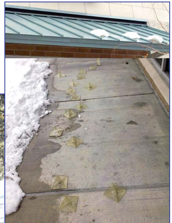
Photo 2 – These plastic snow guards fell to the ground because the adhesive did not bond properly.
