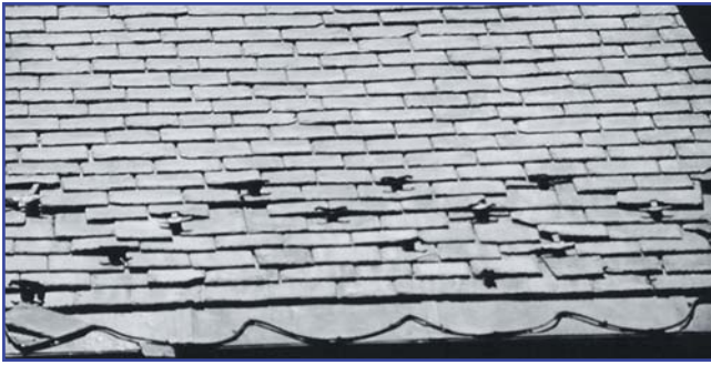
Photo 3 – This snow retention system was not engineered for some variable of the project that caused it to fail.
