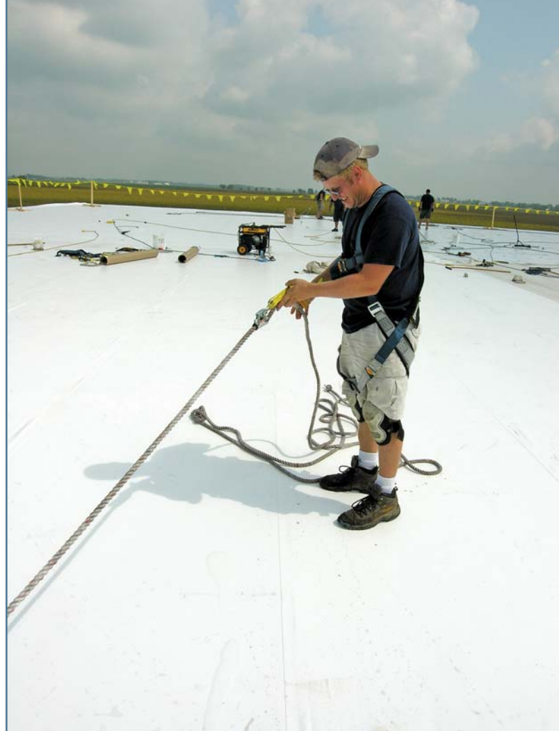
Photo 2 – The objective of SPRI’s field study was to examine roof systems using highly reflective membranes in heating climates. (Photo courtesy of Duro-Last Roofing Inc., Saginaw, MI.)
