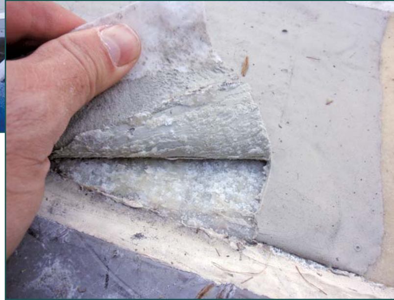
Figure 14 – Substrate failure when deteriorated masonry is not prepared properly.
