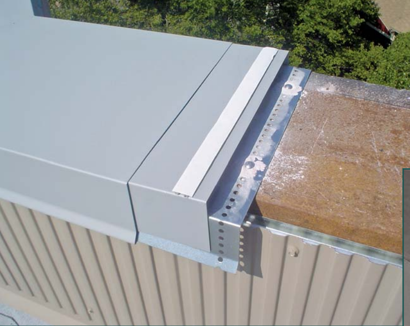
Figure 11 – Coping assembly installed over repointed masonry copings. Note: Concealed splice plate is 12 in. overall, and butyl tape is installed only on horizontal portions.
