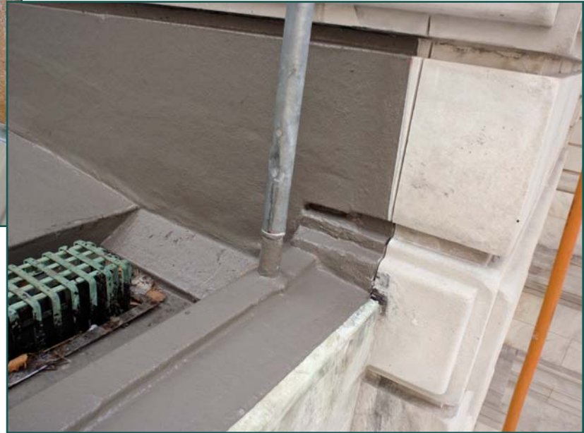
Figure 12 – In-progress detail of self-terminating liquid membrane terminating 1 in. back from coping edge. Membrane continues up cheek wall where the cut reglet detail is visible.
