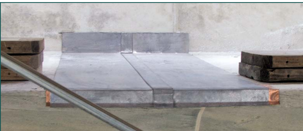
Figure 9 – Flat marble ledge covered with lead-coated copper; connections made with “drive cleat” at seams.
