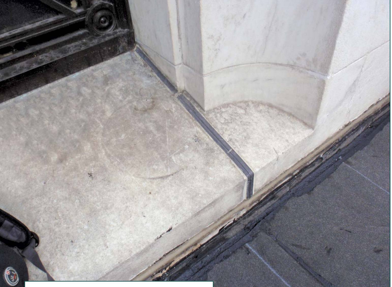
Figure 7 – Transition between up-facing head joint and weathering bed joint lead T caps.
