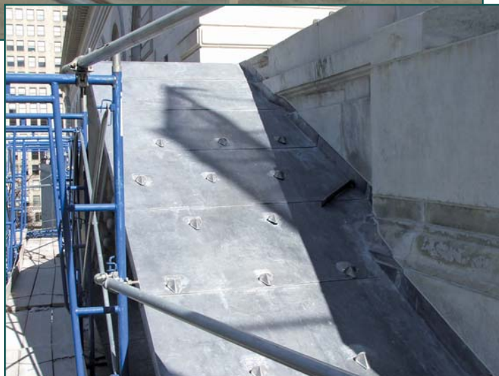
Figure 10 – Inclined marble pediment clad with lead-coated copper; all seams loose-locked.
