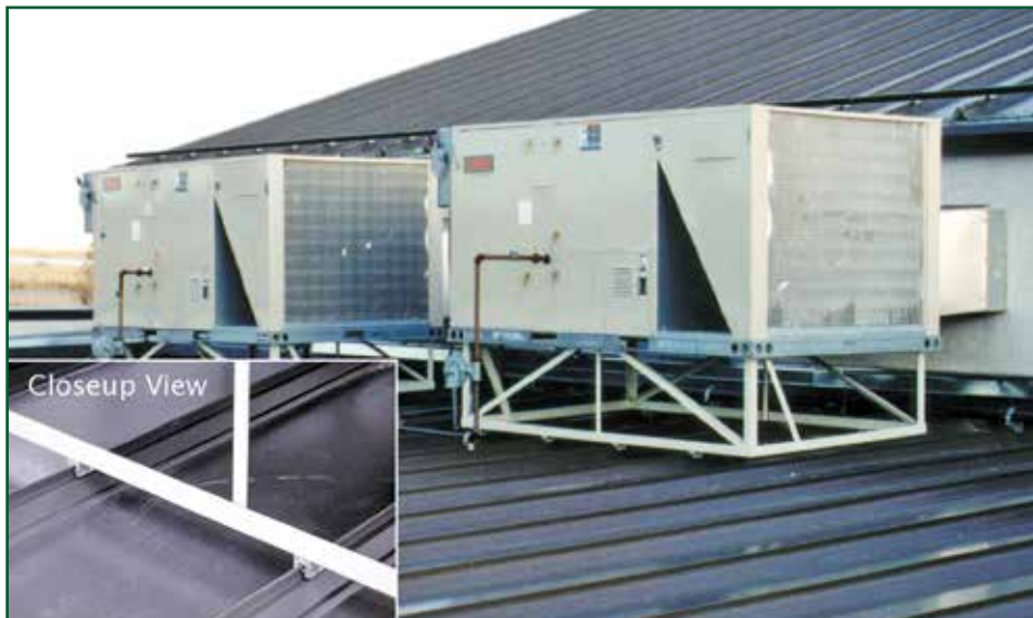
Figure 6 – Frame-mounted HVAC units using seam clamps that avoid roof penetration.
