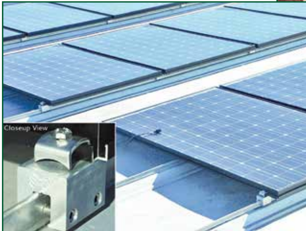
Figure 2 – Seam clamps have made rooftop mounting so simple and cost-effective that metal roofing is now the preferred roof type for mounting photovoltaic solar arrays. Close-up of PV panels with shadow (close-up view of clamp attachment is inset to lower left corner).
