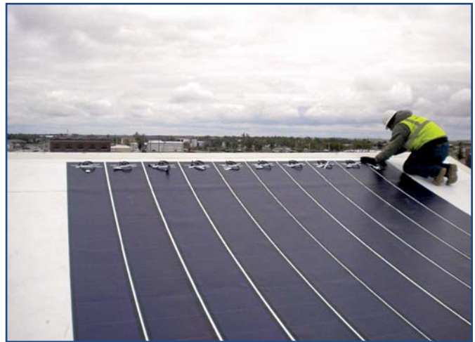
Dark-colored, thin-film PV systems may also contribute to accelerated heat aging of TPO and PVC. In this situation, the roof consultant's safest choice may be a high-performance TPO membrane designed for solar applications.
