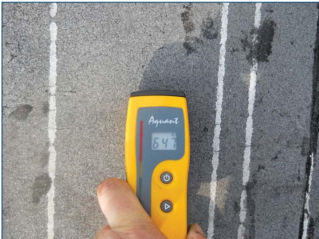
Photo 15 – Elevated moisture identified in the coverboard underneath a built-up roof.
