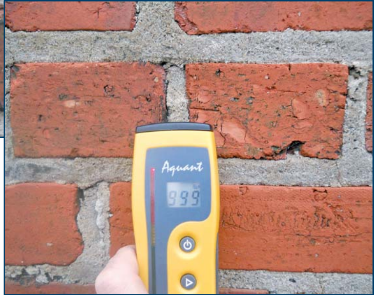
Photo 6 – High (red) reading on mortar.
