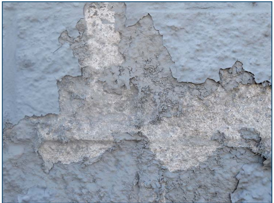
Photo 1 – Moisture in the substrate at the time of application or moisture intrusion months or years later is destructive to most coating systems.
