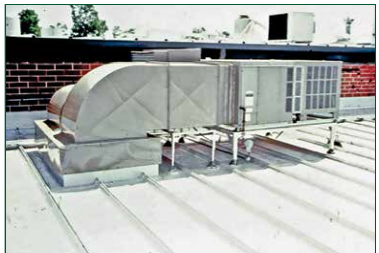
Figure 5 – Frame-mounted HVAC unit using pipe supports extending down to the building structure and flashed through the roof using rubber pipe flashings.
