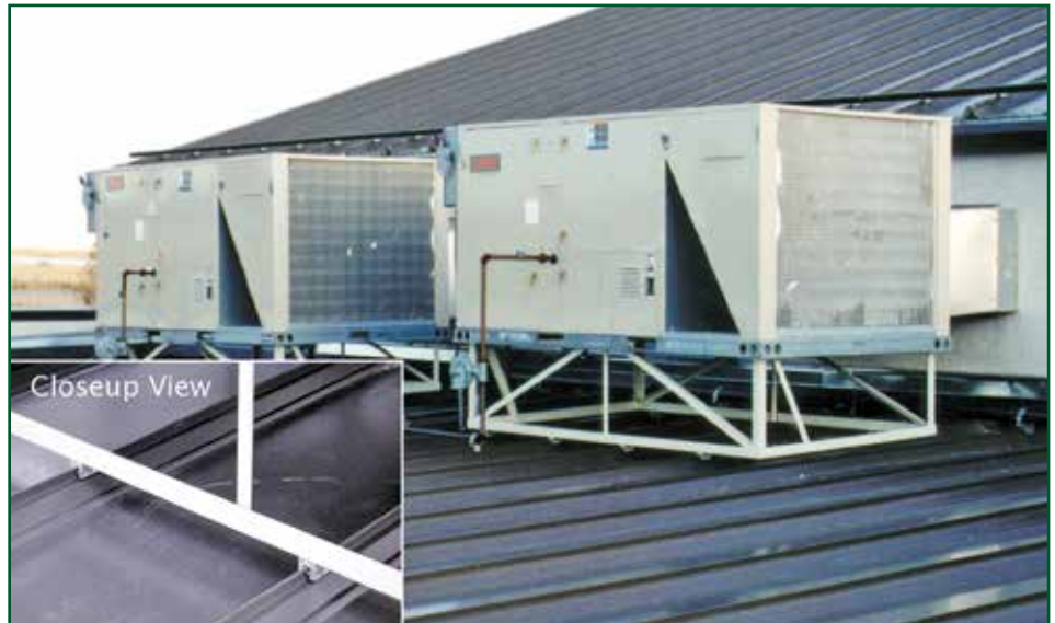
Figure 6 – Frame-mounted HVAC units using seam clamps that avoid roof penetration.
