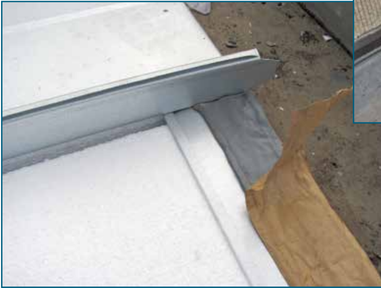
Figure 8 – Vertical-rib panel on triple-bead tape seal over eave trim over 16-gauge offset cleat.
