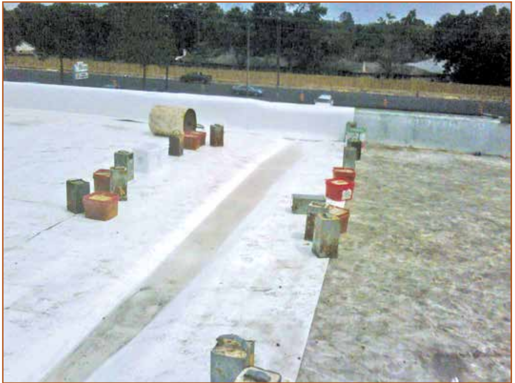
Photo 4 – Water accumulation on depression at tie-in.
