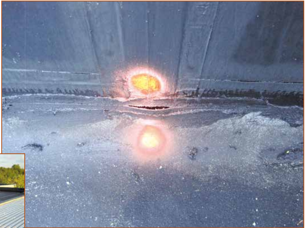
Photo 6 – Disbonded felts along parapet wall.
