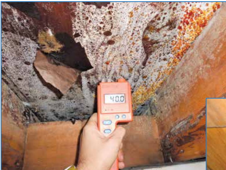
Photo 1 – Very high moisture content. The surface of the wood was wet.
