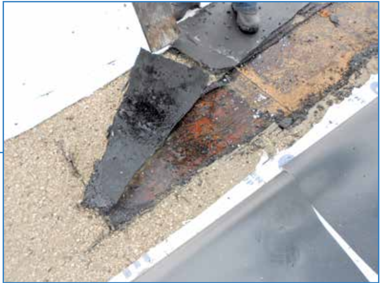
Photo 4 – Moisture was accumulating between the roof deck and the BUR.
