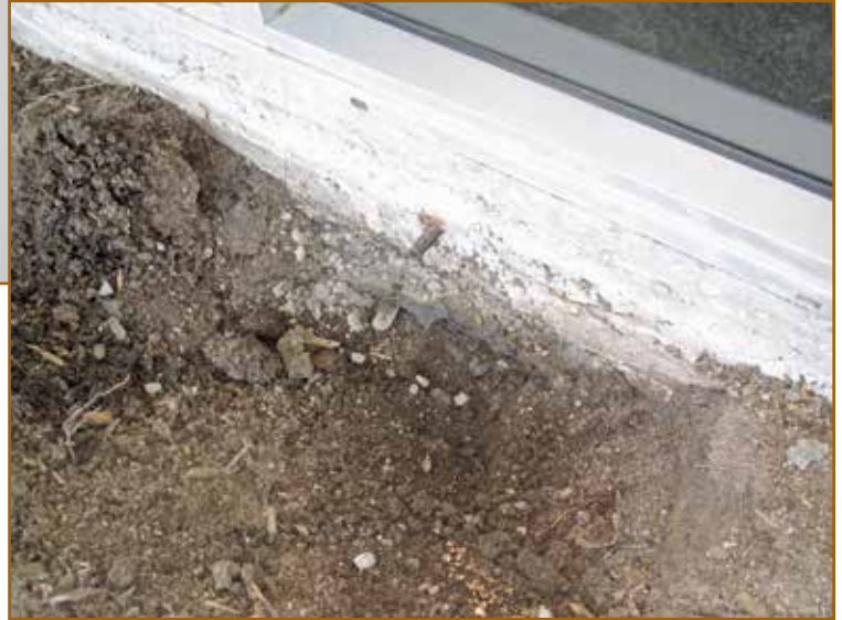
Photo 11 – Soil in planter directly abuts the granular subgrade under the concrete slab. The punctured polyethylene vapor retarder is visible under the corroded rebar.
