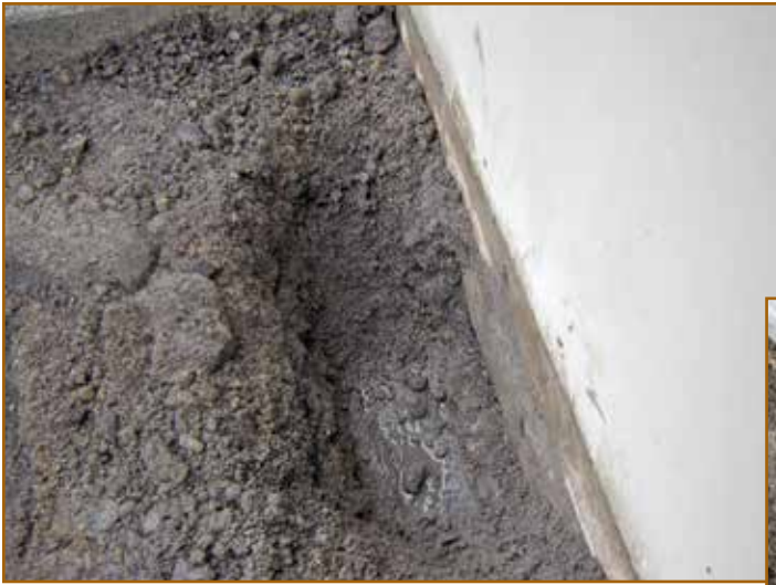
Photo 10 – Test cut C-3 at sidewalk: Water began seeping outward from under the concrete tilt-up panel.
