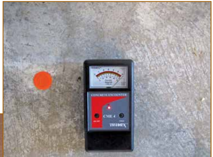
Photo 5 – Electrical impedance confirms floor slab is saturated.
