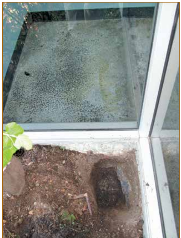
Photo 15 – The pour strip (or pour-back strip) 21 within Unit 12 was saturated. The planter drains under the slab via the LTS pad.
