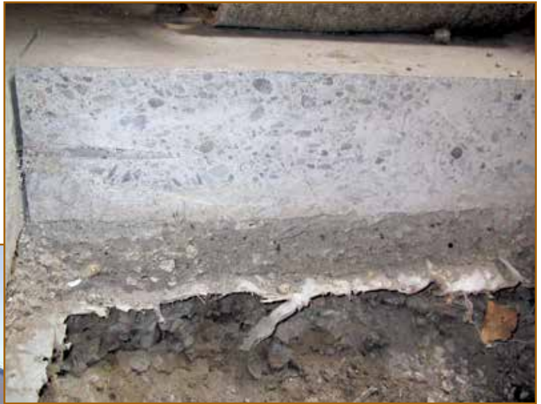
Photo 7 – Test cut C-1 exposes the overlap joint of the 10-mil polyethylene vapor retarder.
