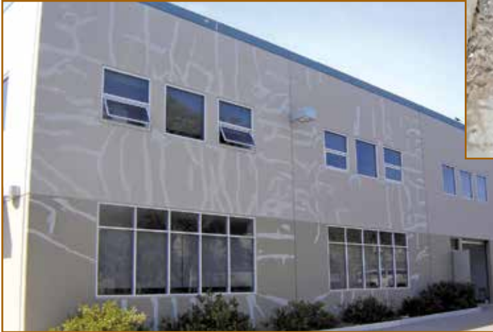
Photo 6 – Widespread cracking of concrete tilt-up panels was an exacerbating source of water infiltration.
