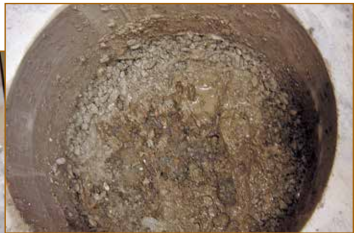
Photo 9 – Test core C-2: Pooling water was found directly under the floor slab.
