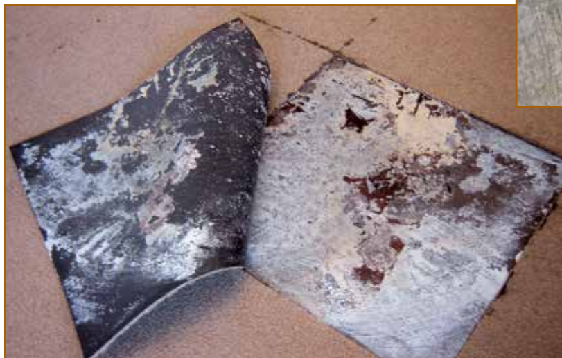
Photo 4 – Latex adhesives are emulsified and deteriorating, creating smelly IAQ problem.
