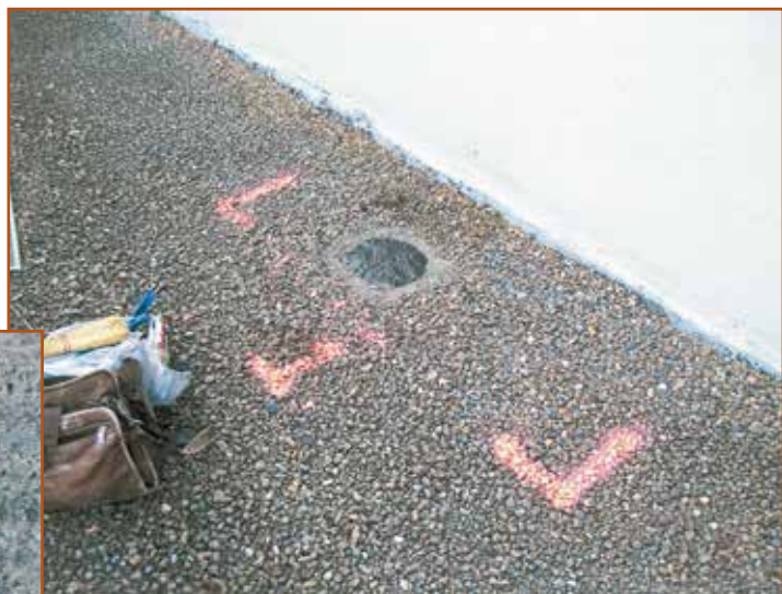
Photo 21 – View of anomaly of wet perlite under BUR.
