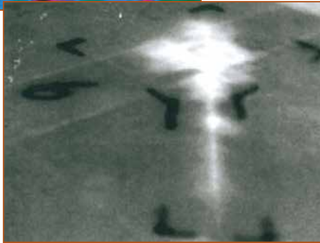
Photograph 4: View of wet insulation occurring along joint between ISO boards (gray contrast).
