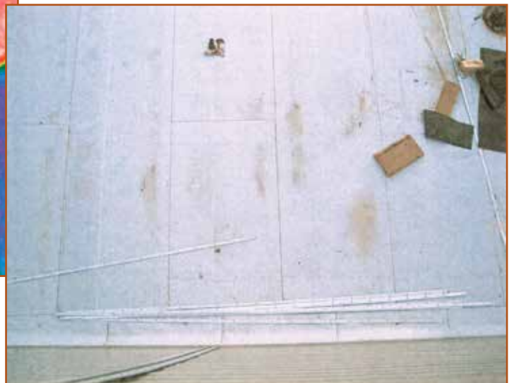
Photo 11 – View of soiled areas of white-surfaced modified-bitumen cap sheet.
