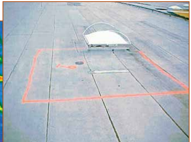
Photograph 6: View of anomaly of wet ISO under modified-bitumen membrane.
