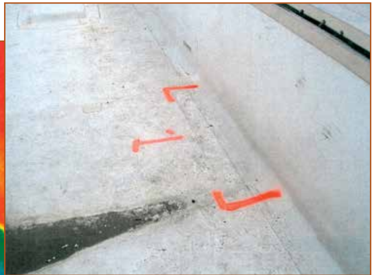
Photograph 16 – View of anomaly location of water in TPO base flashing.
