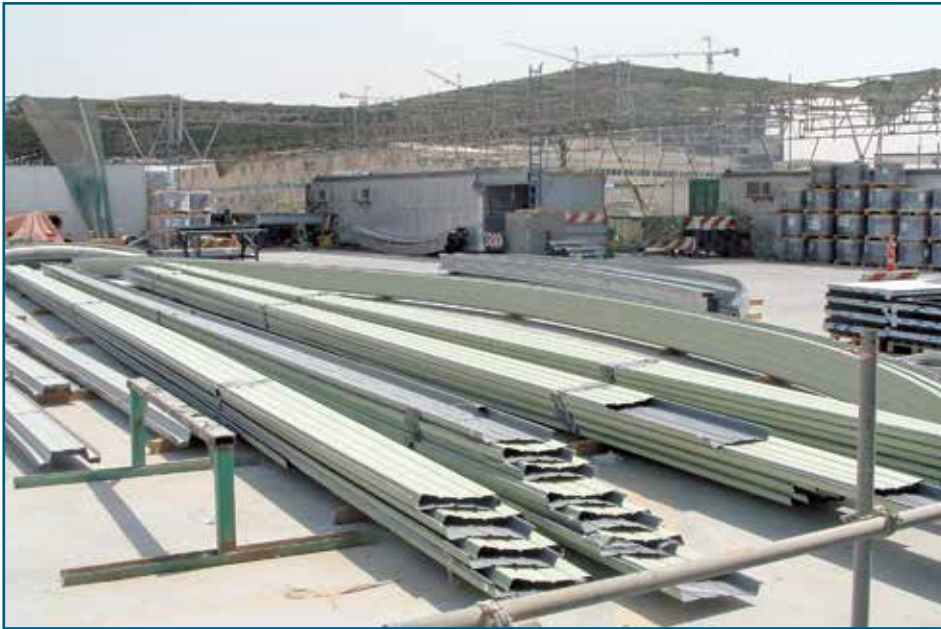
Figure 5 – Part of the Dubai Terminal on-site temporary factory with stocks of finished product in the foreground.
