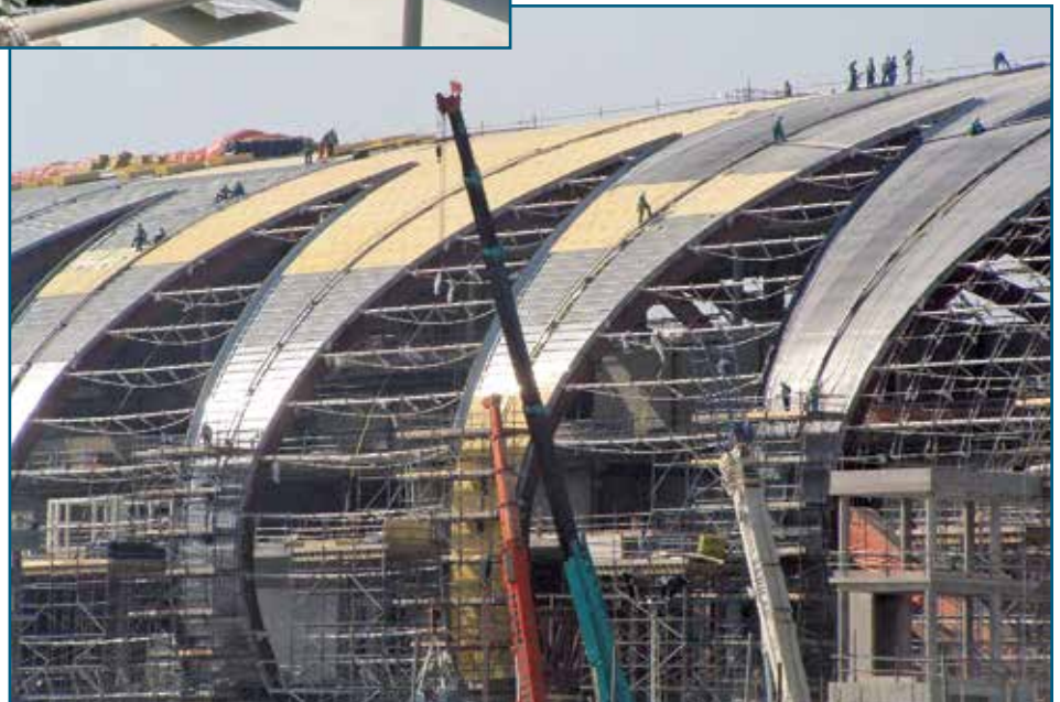
Figure 6 – Crane lifting secondary components to the roof level. Special on-roof support platforms were required.
