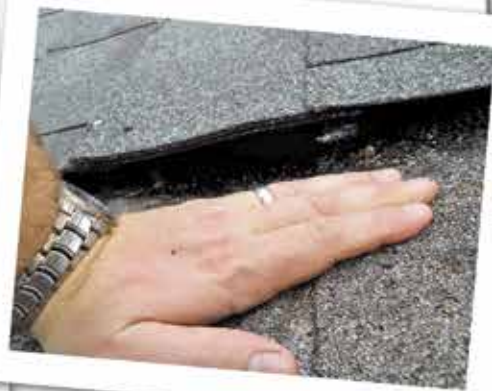
Photo 5 - Pressing next to the laminate shingle exposed the interior of the attic to view.
