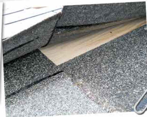
Photo 7 - No underlayment under the new three-tab shingles.
