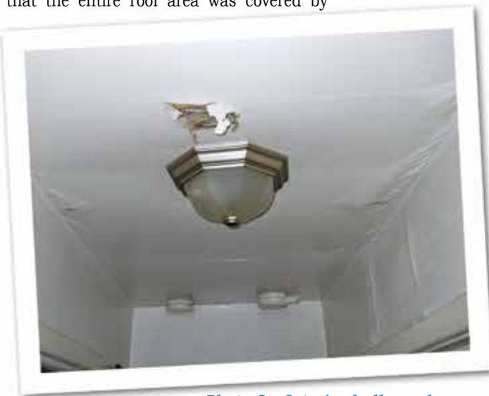
Photo 2 - Interior hallway damage.
