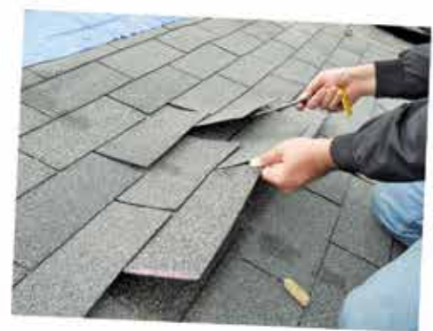
Photo 6 - Improper nailing of new three-tab shingles.
