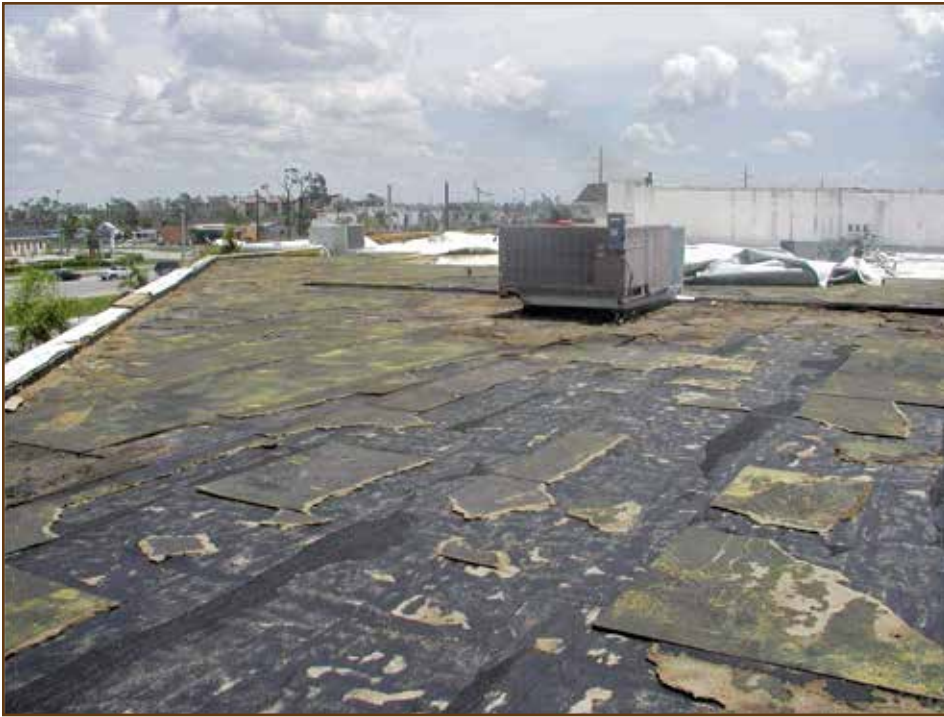
It is likely that FM Approvals believes its changes to FM 4470 will reduce insurance risk and provide greater safety factors on FM-insured buildings. Despite the roof damage shown here after a Florida hurricane, the integrity of the roof deck has not been compromised. (Photo courtesy of SPRI.)
