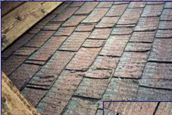
Photo 15 – Close-up of cracking granule surfacing on the west slope of the lower north end.
