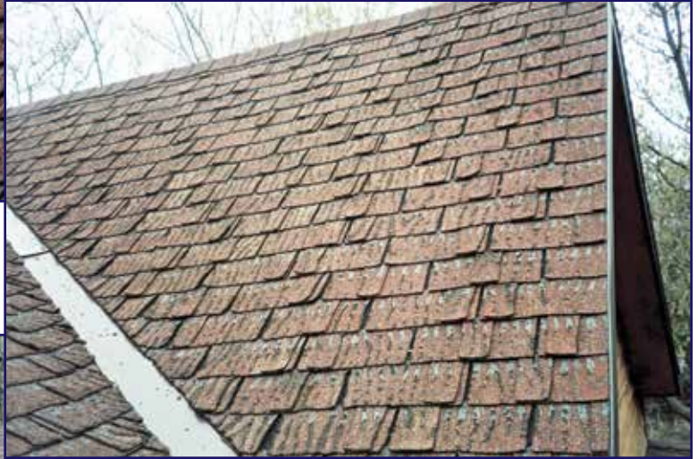
Photo 9 – View of NE valley and shingles on north end of south slope. No impact marks on metal valley.
