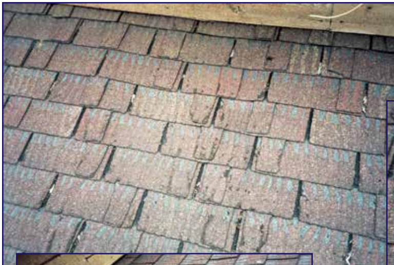
Photo 13 – Close-up of cracking granule surfacing on the east slope of the lower roof.
