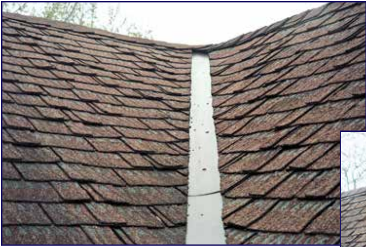
Photo 8 – View of SE valley on upper main roof. No impact marks on metal.
