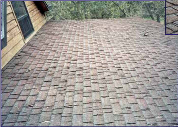
Photo 10 – View of deteriorated shingles on east lower slope.
