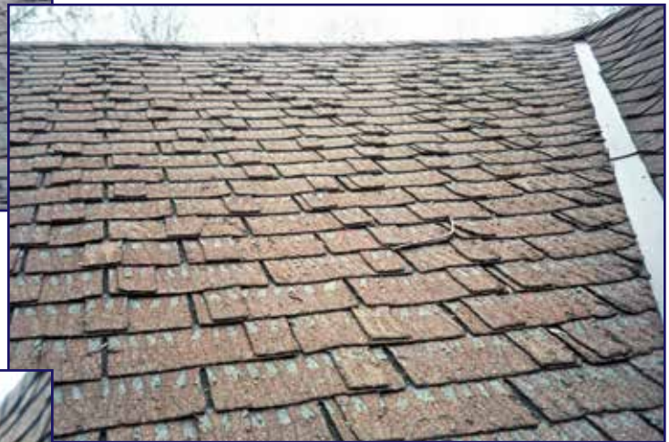
Photo 11 – View of deteriorated shingles and metal valley. No impact marks on metal on north end of upper west-side roof.
