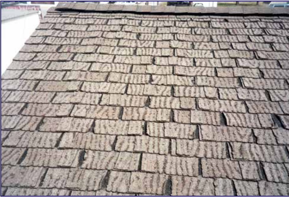
Photo 6 – West slope, cracking of granule surfacing.
