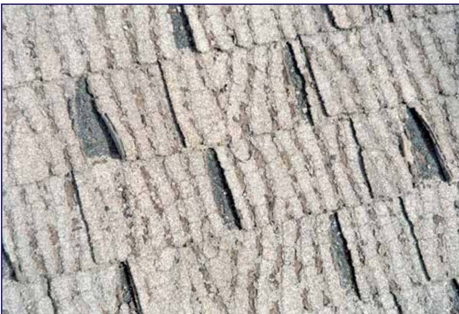
Photo 5 – West slope, close-up of cracking of granule surfacing on shingles.
