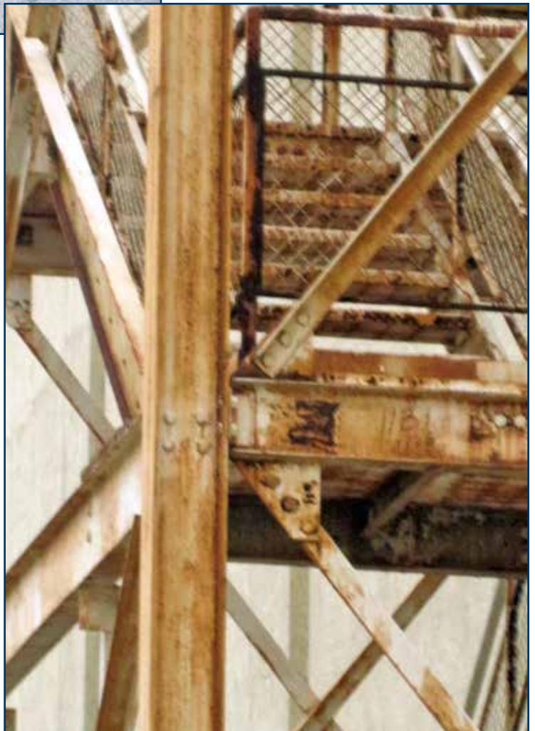
Photo 4 – Corroded fire escape.
