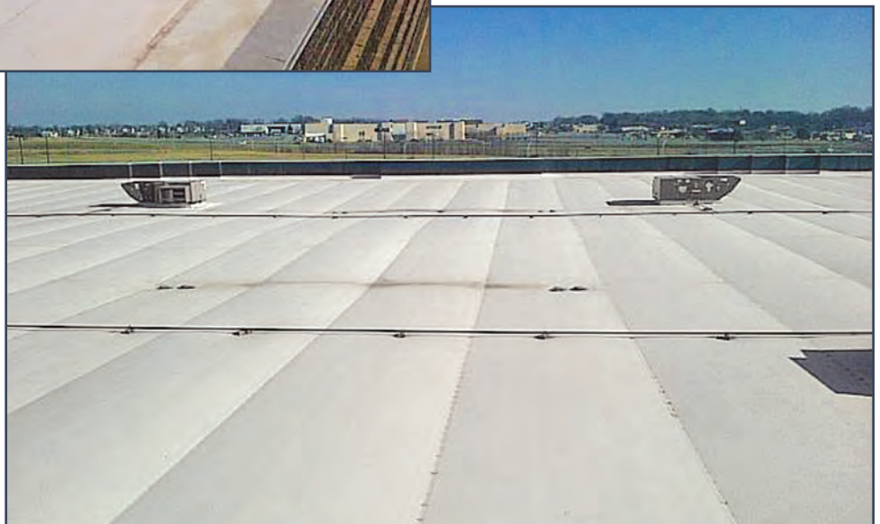
Figure 4 – Positive pressure in this facility’s mechanical system causes membrane to billow.
