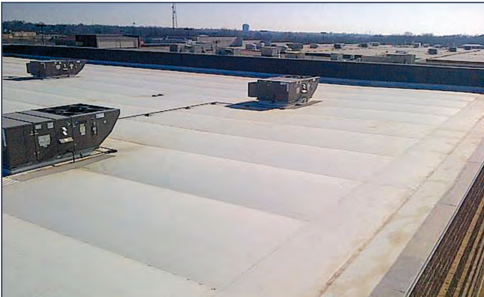
Figure 3 – Billowing, mechanically fastened roof system over a pressurized building.
