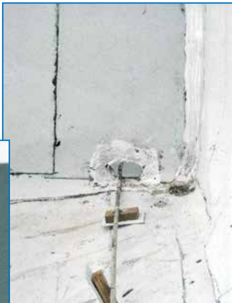
Figure 3 – Roof base flashings covering overflow scupper drains of collapsed roof.
