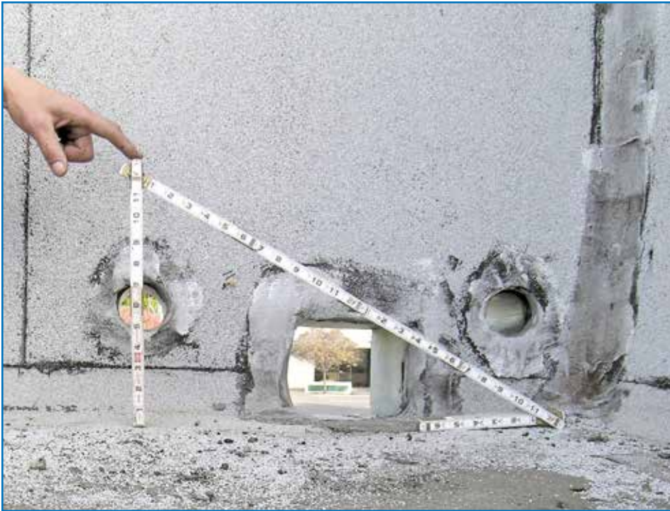
Figure 4 – Scupper drain and scupper overflows of collapsed roof after reconstruction. Note: They were reconstructed the same size.
