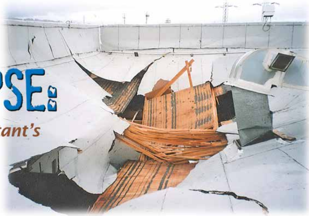
Figure 1 – Roof collapse after very intense but less-than-code-level rain.
