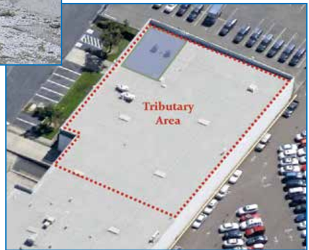
Figure 5 – Aerial view of roof overlaid to show collapsed area (blue) and scupper drain tributary area (dashed red line). Image from Google Earth Pro.
