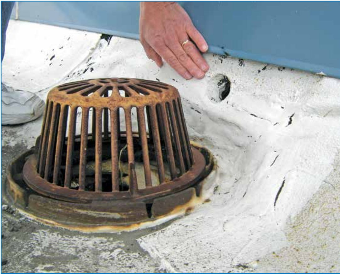
Figure 6 – One-and-a-half-inch diameter overflow “hole” about 3.5 in. above a 5-in. drain.
