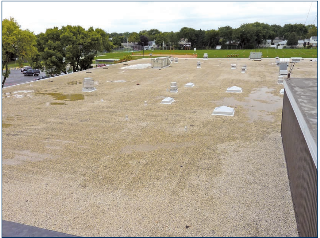
Photo 1 – Coal-tar roof with ponded water.
