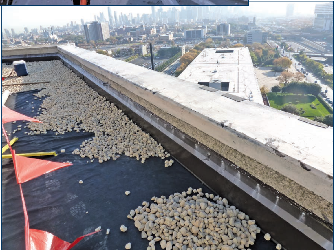
Photo 7 – A PRMA roofing membrane with filter fabric and ballast rock being installed.
