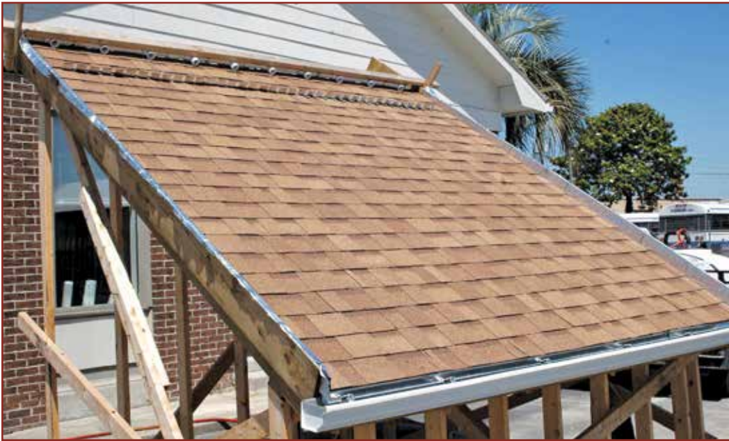
Photo 2 – Overview of the test stand showing the water distribution manifold along the ridge and the 5K Ogee gutter along the eave.
