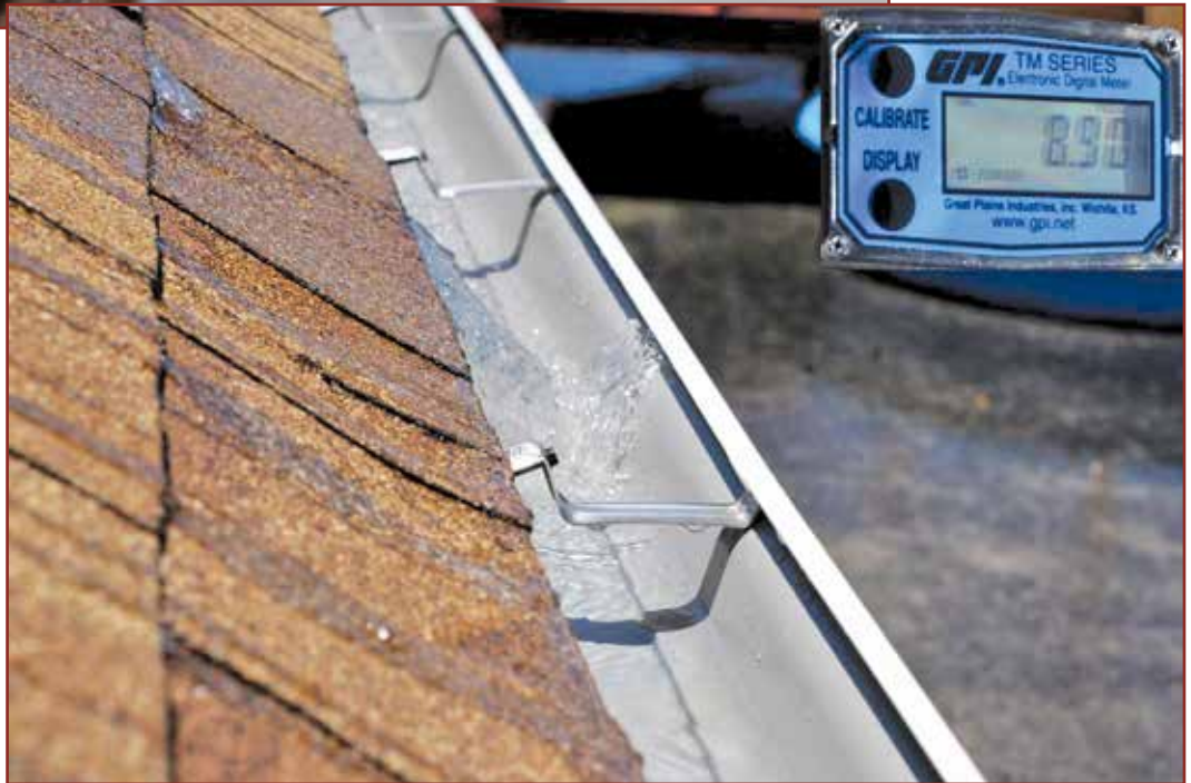
Photo 8 – At 8.9 gpm, the momentum of the flow was sufficiently low for the water to be retained by the gutter.
