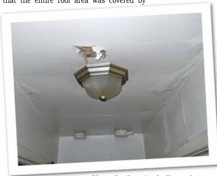
Photo 2 - Interior hallway damage.
