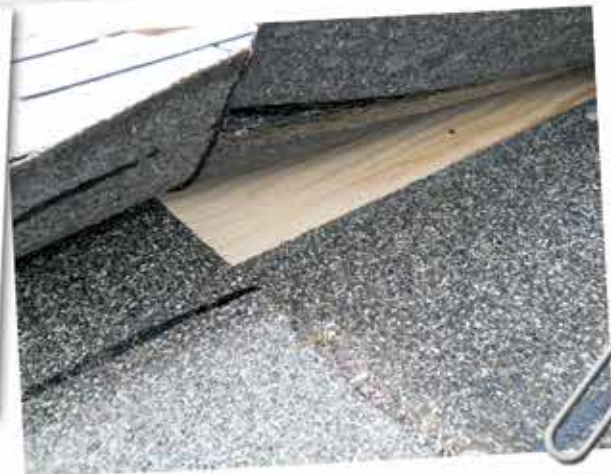
Photo 7 - No underlayment under the new three-tab shingles.
