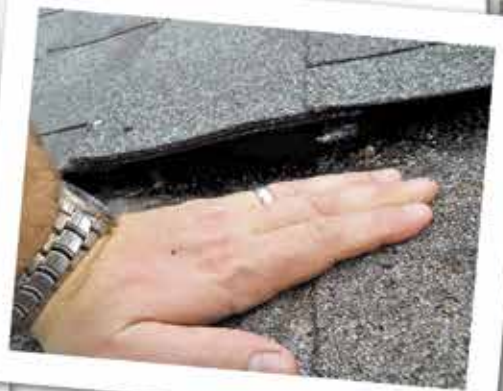
Photo 5 - Pressing next to the laminate shingle exposed the interior of the attic to view.
