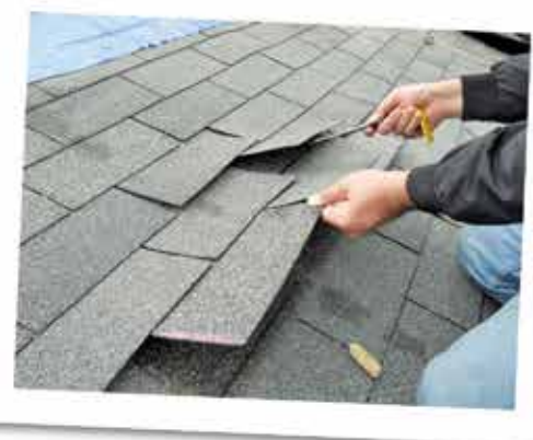
Photo 6 - Improper nailing of new three-tab shingles.
