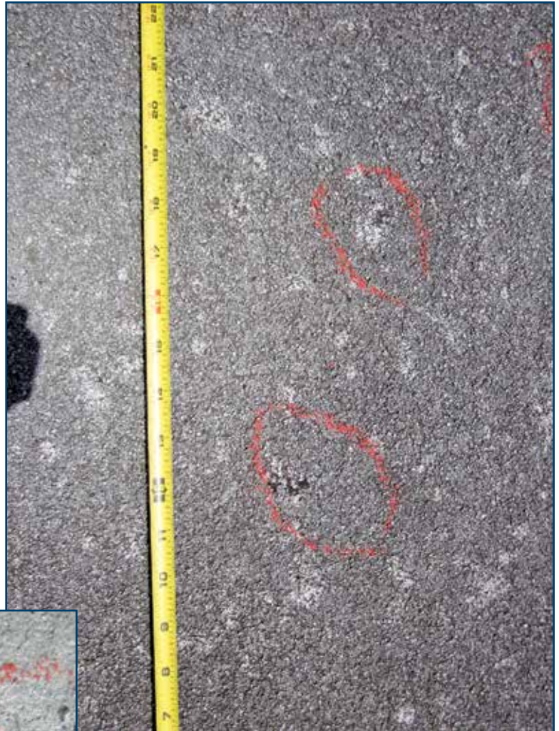
Photo 4 – Overview of hail strikes on a granule-surfaced cap sheet. The two worst hail strikes are circled. Each showed granule loss and felt soft or “bruised.” The additional white marks are also hail strikes, but not as severe. Removal of the oxides from the granules leaves a clean spot or “splash mark.”
