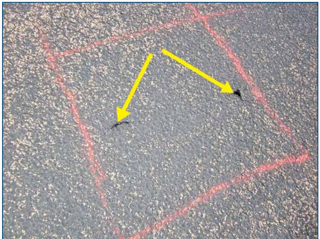
Photo 1 – Complete fracture of low-slope bituminous roof membrane from hail strikes. Membrane was installed over fiberglass board insulation, a less-dense coverboard in comparison to a gypsum substrate.
