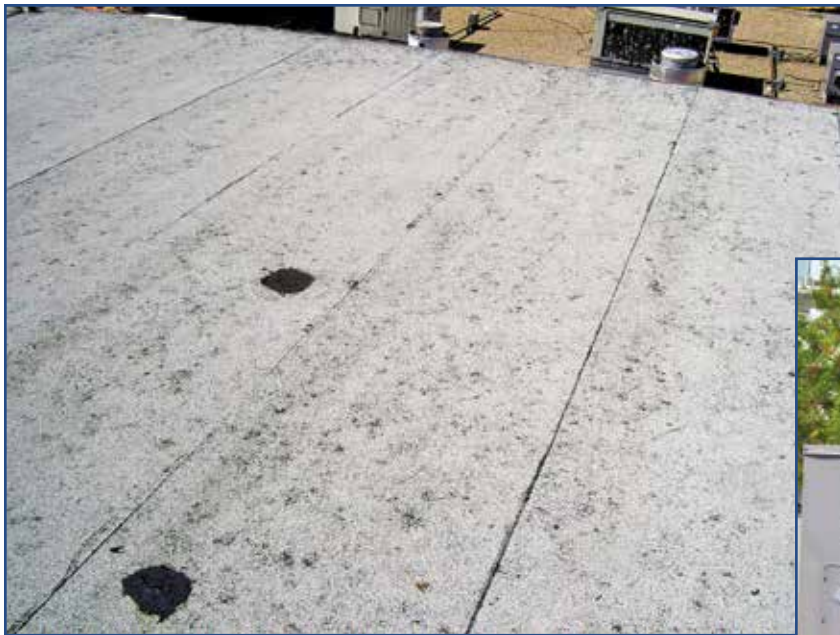
Photo 3 – Hail damage to modified roof system.
