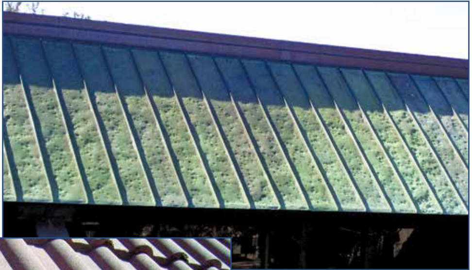
Photo 5 – Damage to copper standing seam.
