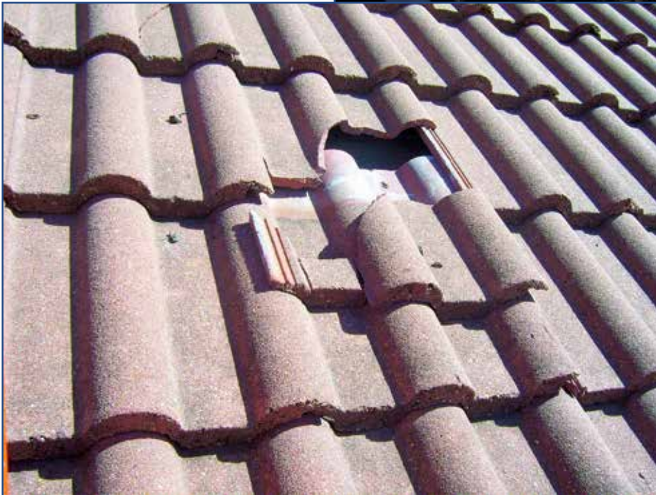
Photo 6 – Damage to concrete tile.
