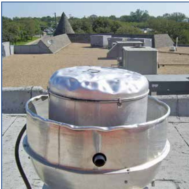
Photo 1 – Damage to exhaust fan at modified bitumen roof system.
