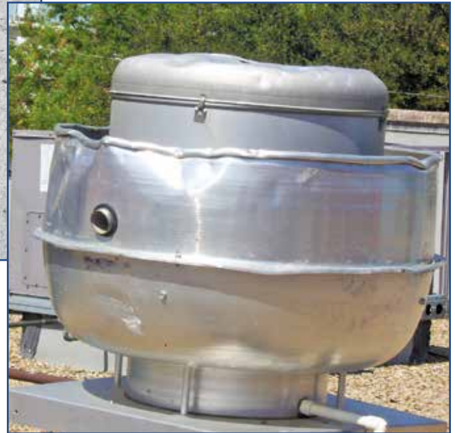
Photo 4 – Damage to exhaust fan at aggregate surfaced BUR.
