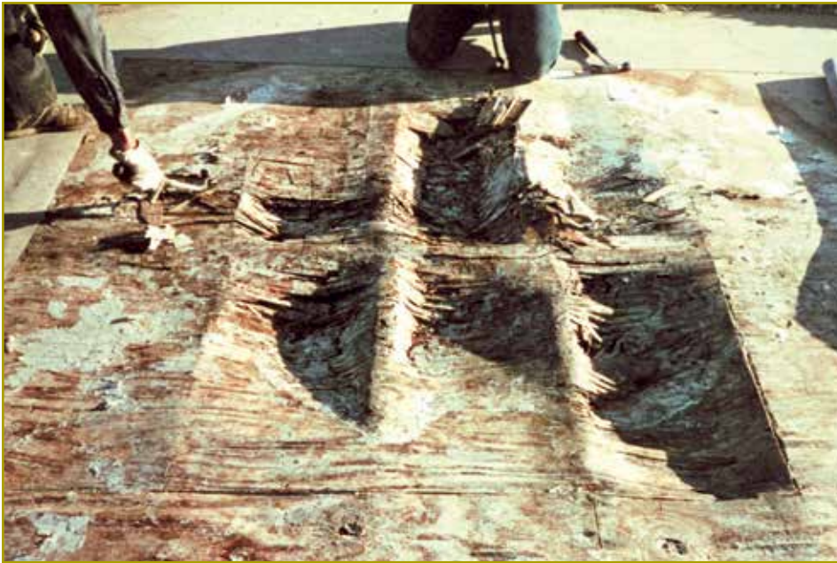
Figure 2 – Severe deterioration caused by water vapor migrating up through the ceiling of a laundry room.
