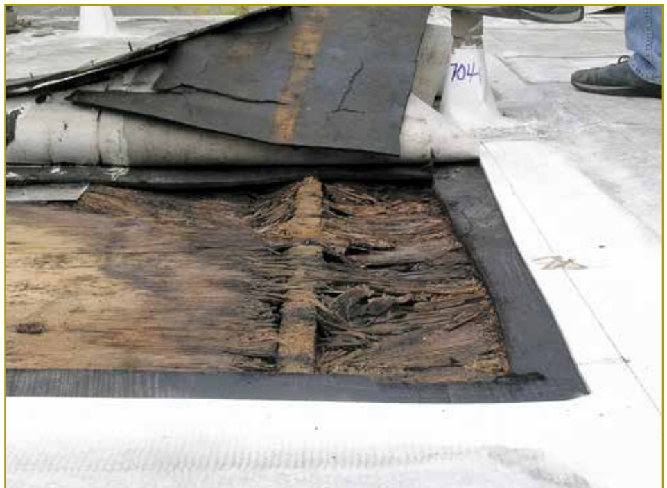
Figure 1 – Severely deteriorated plywood a few years after replacing an old cap-sheet BUR with a white single-ply roof.
