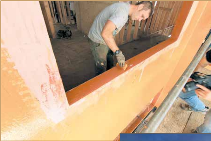
Figure 7 – An installer seals a rough opening with an STPE-based flashing at an under-construction passive house in Yamhill County, OR. The builders chose the fluid-applied flashing because of demonstrated performance in stopping air leaks through the building envelope. Photo courtesy of Hammer and Hand.
