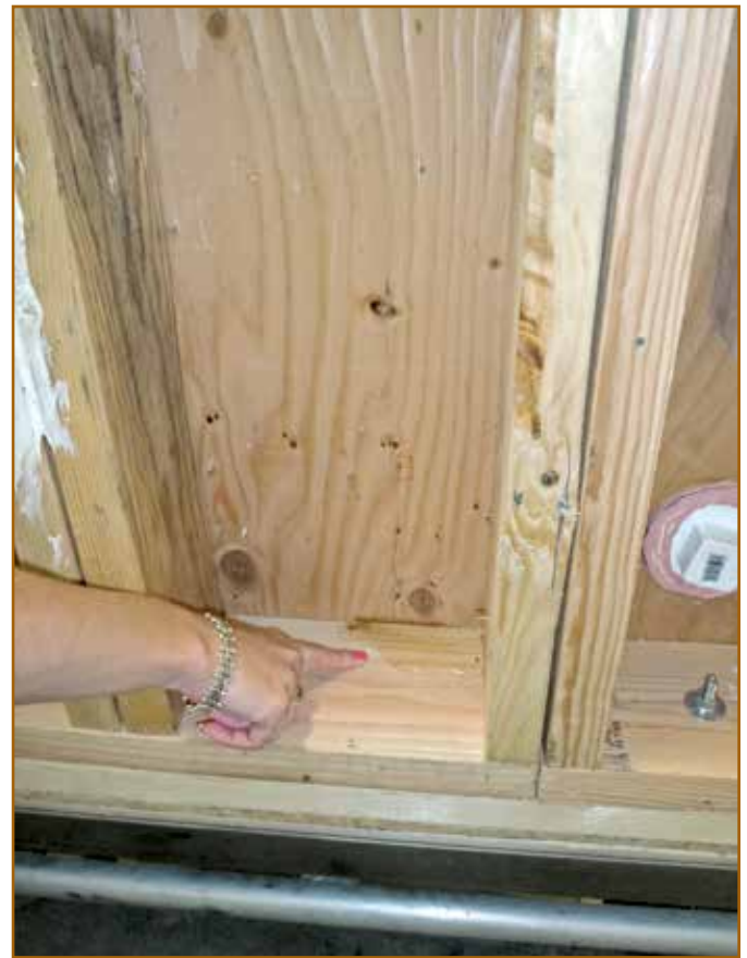
Figure 6 – An inspector points to where air pressure, simulating wind-driven rain, has forced a leak in a wall assembly mock-up during testing in the Design Verification Test Chamber. Photo courtesy of PROSOCO.
