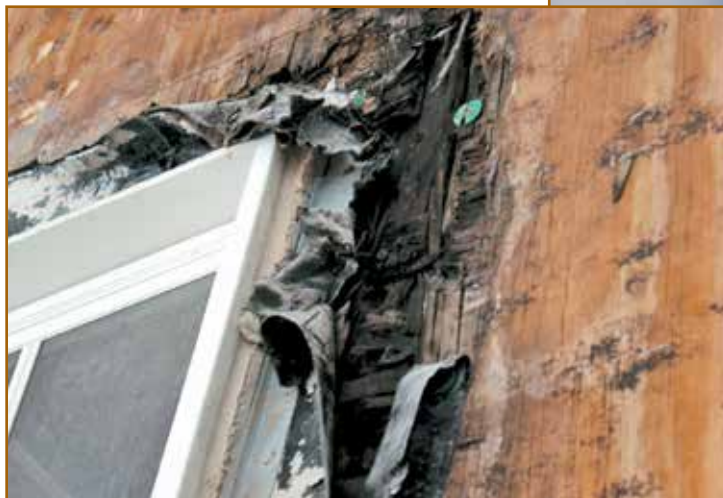
Figure 1 – This rotted plywood from a vapor-impermeable peel-and-stick that trapped moisture is typical of what repair contractor Tatley-Grund, Seattle, finds in water-damaged buildings. They found it counterproductive to repair problems like this with the same methods that they felt caused the damage to begin with. Photo courtesy of BEI, LLC.
