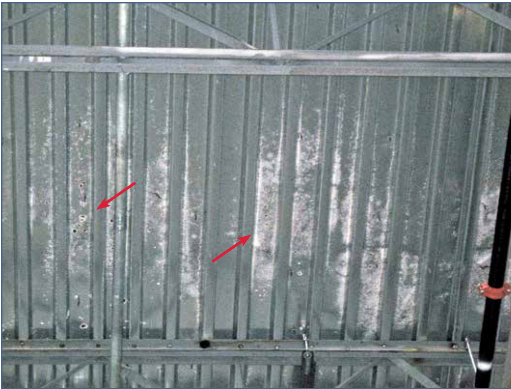
Figure 3 – Small red rust spots (left arrow) and white rust (right arrow) developing on bottom side of roof deck.
