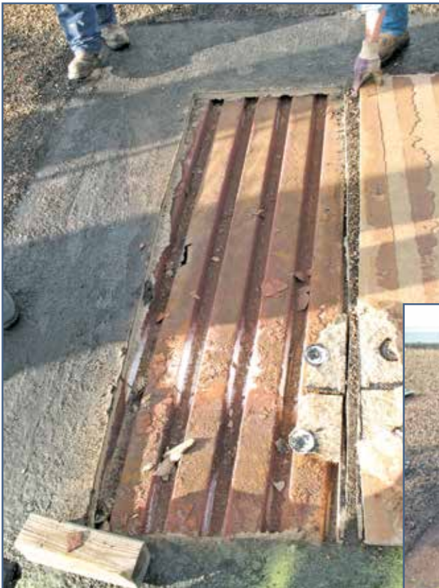
Figure 1 – Roofing membrane and insulation board removed to expose metal decking. Note corrosion occurs at both “peaks” and “valleys” of metal decking.
