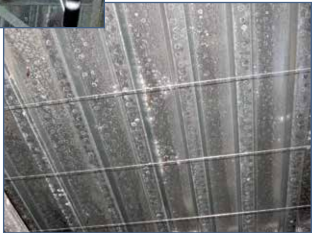
Figure 4 – White rust starting on bottom side of roof deck looks like deposits from water droplets.
