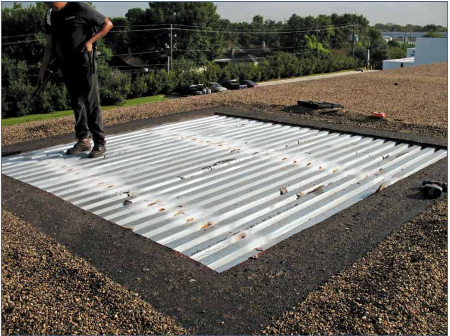
Figure 5 – Lines of white rust on top of metal deck at spot welds.
