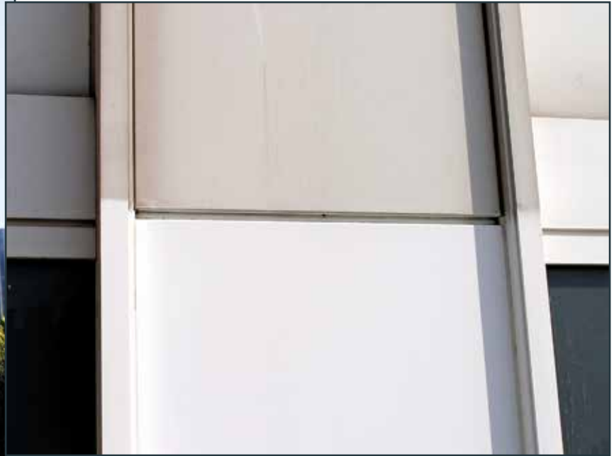
Demarcation between restored and unrestored areas of this clear anodized aluminum building is apparent.
