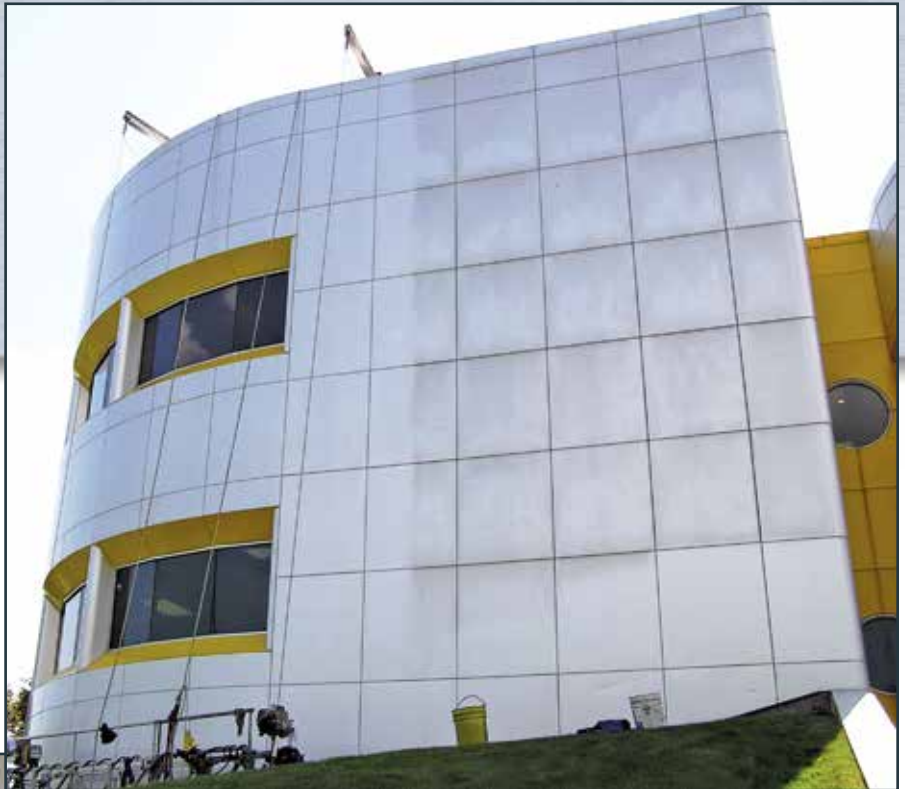
This clear anodized aluminum building in Grand Rapids, MI, is in the process of being cleaned.
