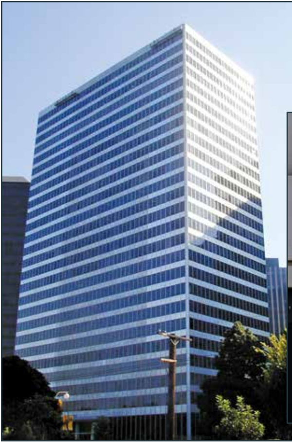
Restoration is progressing from both corners of the façade on this anodized aluminum Century City high-rise.
