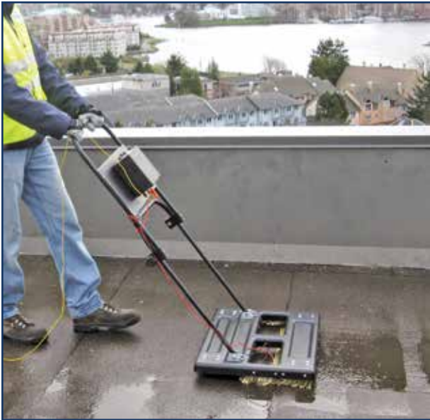
Figure 3 – Scanning deck method of low-voltage testing uses metal chains hanging from the deck instead of a trace wire and probes.
