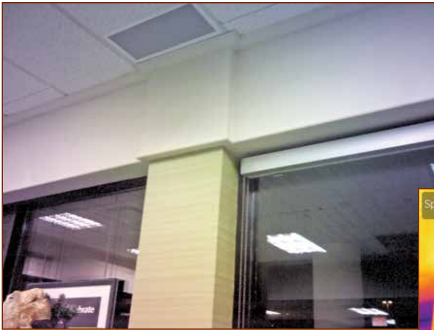
Figure 1 – Visual image of column and window interface at Site 1.
