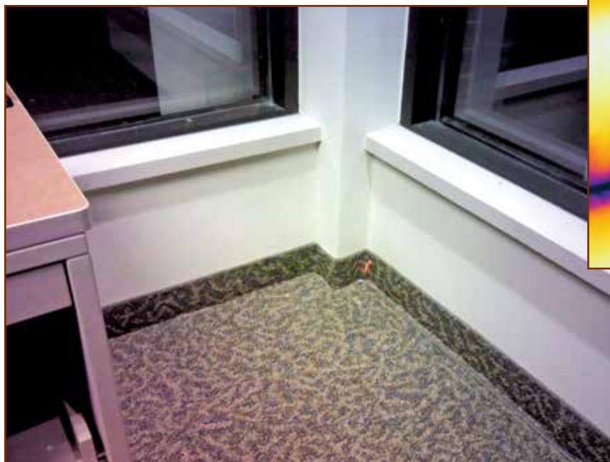
Figure 3 – Visual image of wall with floor interface in corner office at Site 1.
