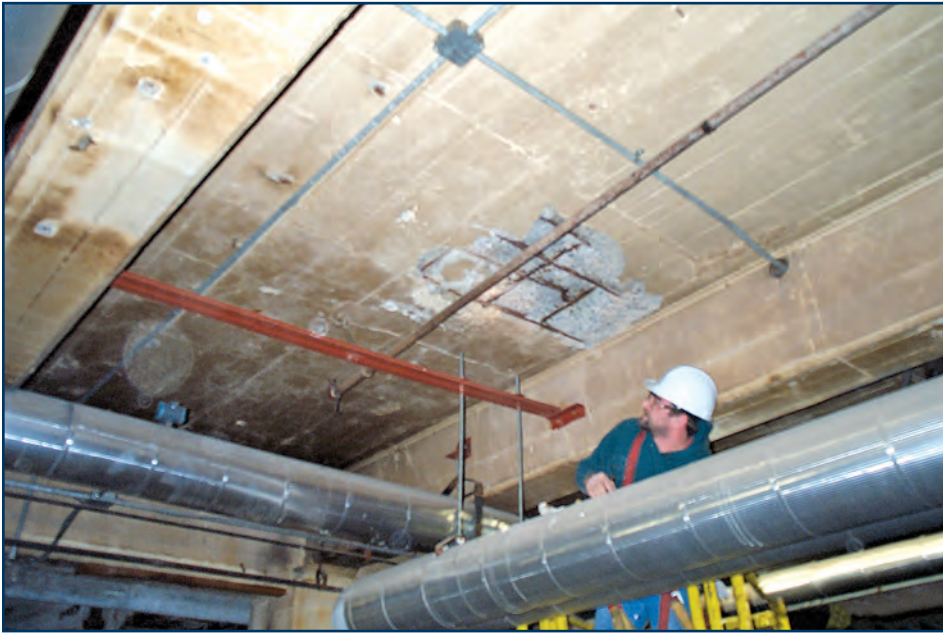
Photo 10 – Spalled concrete caused by expanded corroded rebar. (Photo by Bailey and Son Engineering.)
