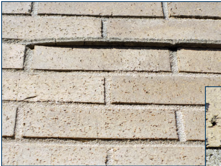
Photo 7 – Mortar expelled by expanded and corroded reinforcement. (Photo by Cris Crissinger.)
