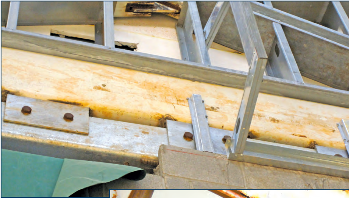
Photo 13 – Corrosion and rust bloom during construction. (Photo by Cris Crissinger.)
