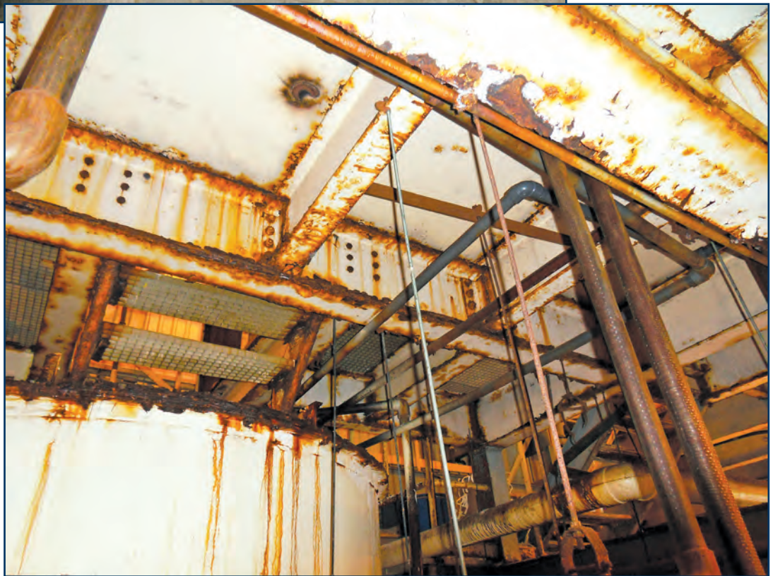
Photo 14 – Structural steel corrosion from protective coating failure. (Photo by Bailey and Son Engineering.)
