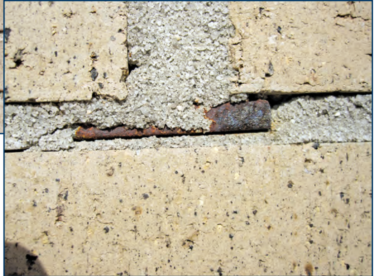
Photo 8 – Exposed masonry reinforcement. (Photo by Cris Crissinger.)
