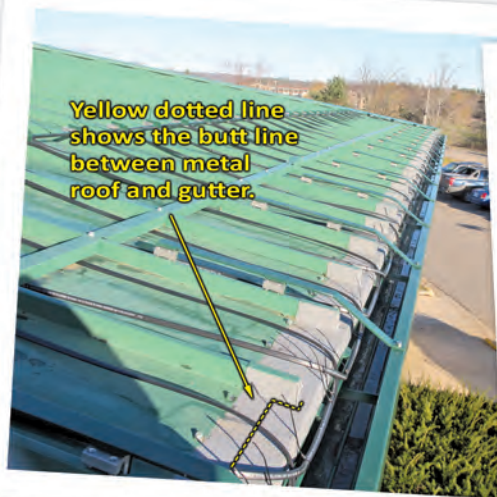
Figure 5 –View of the complete installation of gutter and heating cable.
